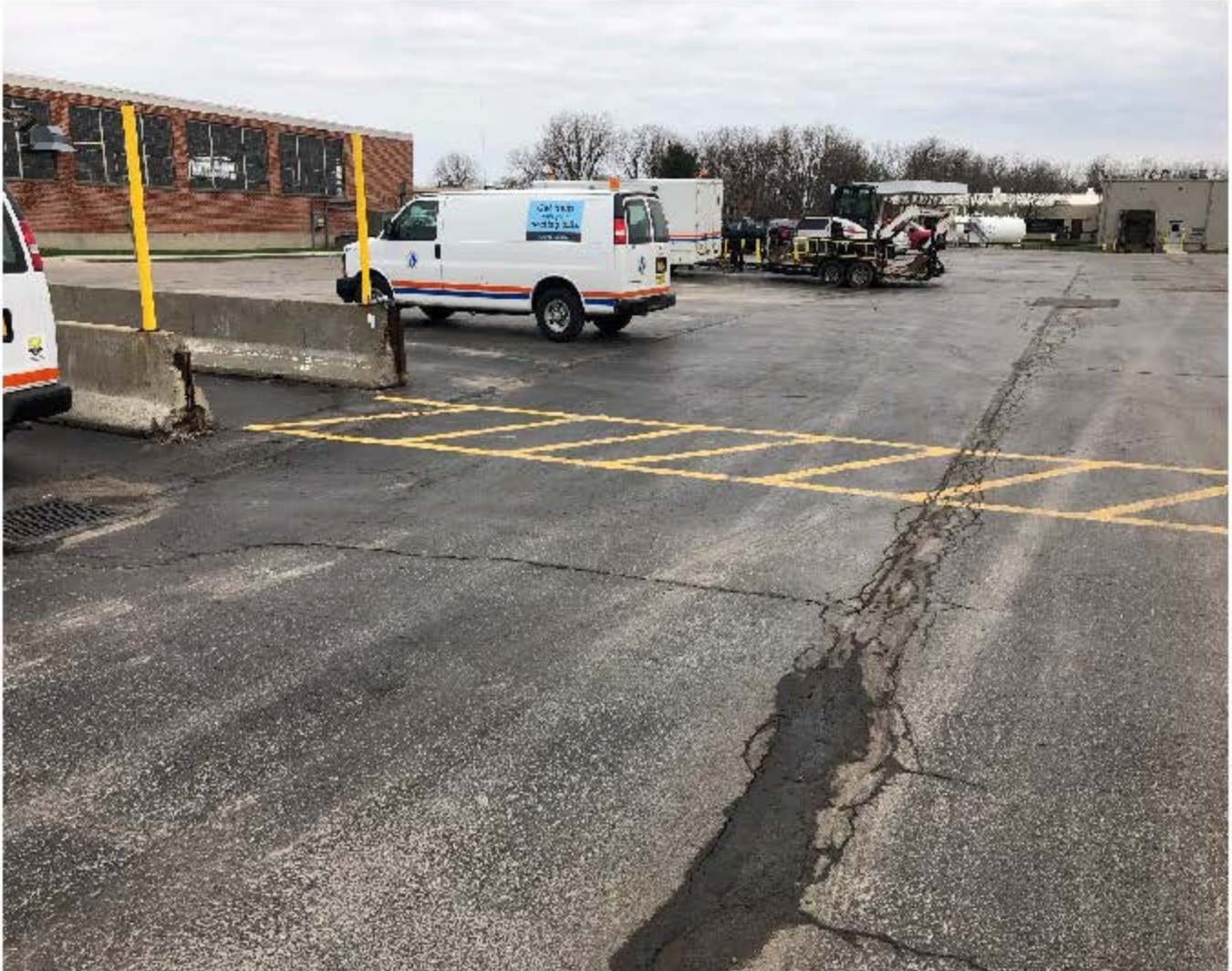
Photo 11. North view of Bldg. 3 East Asphalt Cap (B3EAC) with surface cracks and prior sealing.
