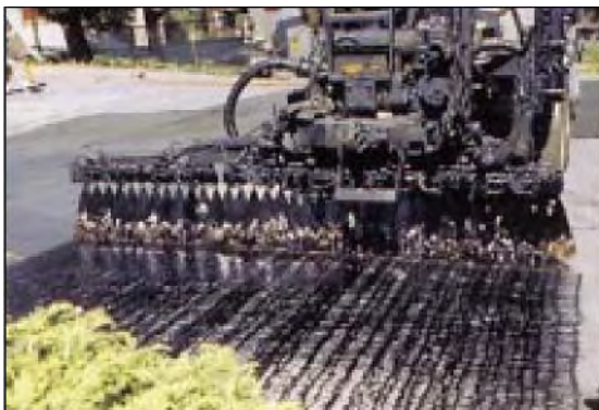
Close-up of streaks of asphalt tack coat. Streaks are unacceptable for the installation of the Petromat system (refer to Part II C of this
