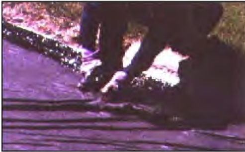
Photograph of wrinkle that requires repair.
