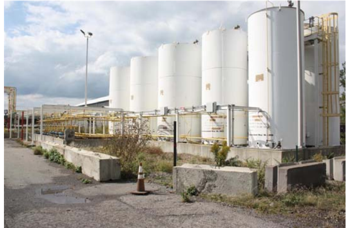
AST Tank Farm
