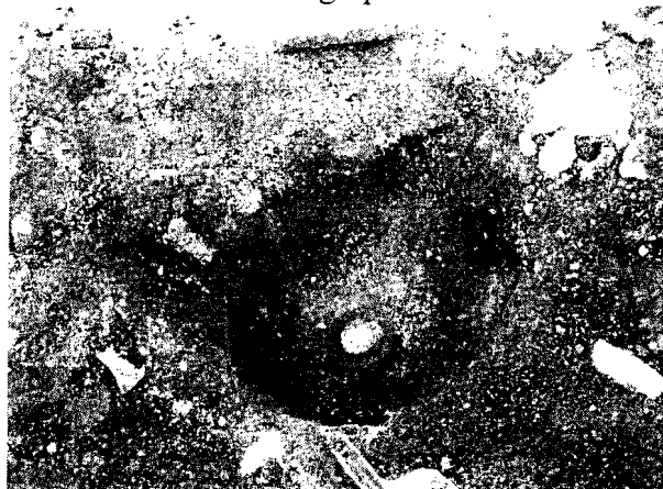
Leaching Pool Cleanout Pipe with Plug
