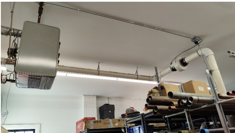
Photograph #105 – View of SSDS fan.
