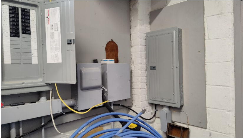
Photograph #103 – View of plumbing warehouse control panels.
