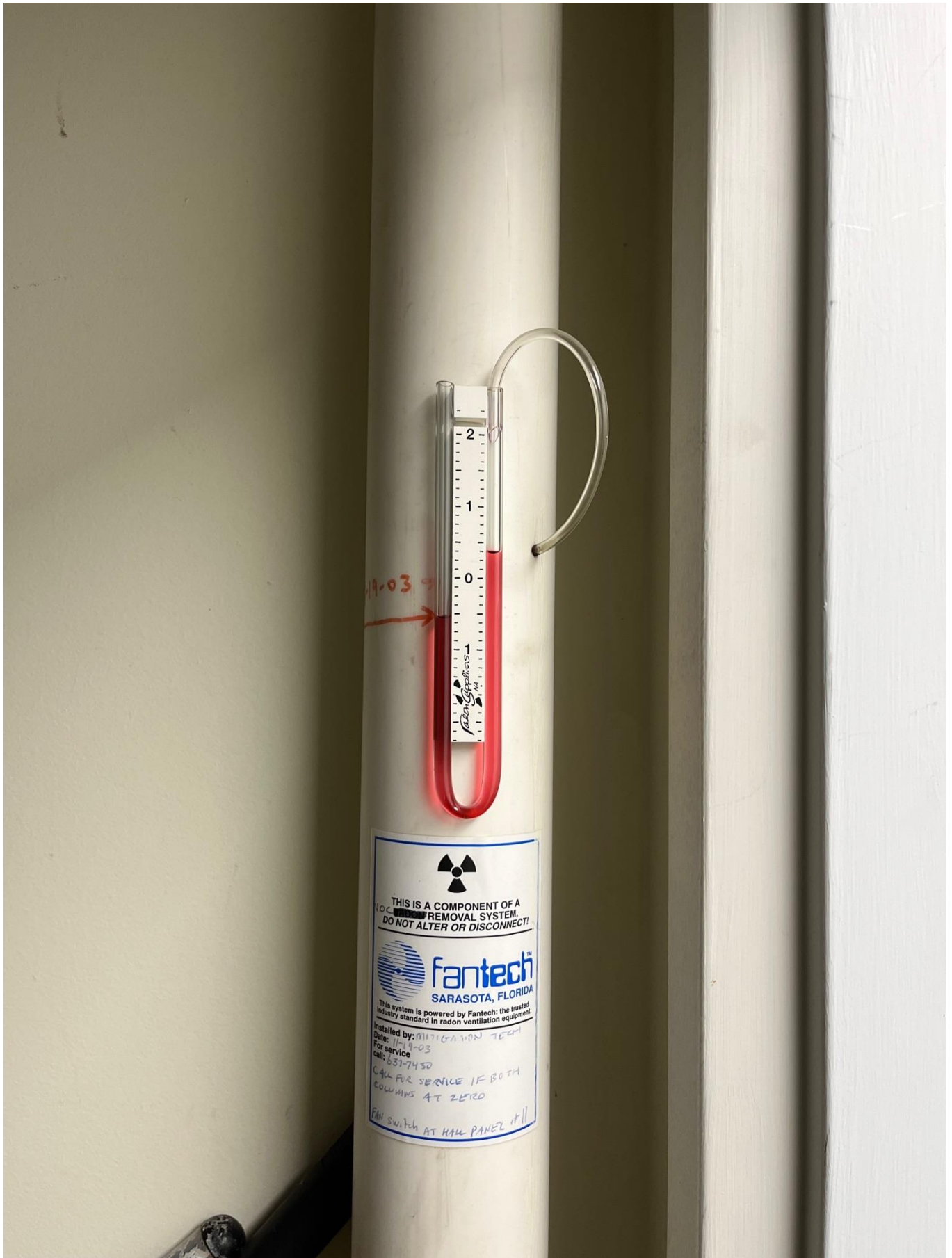
Sub-Slab Depressurization System November 30, 2022
