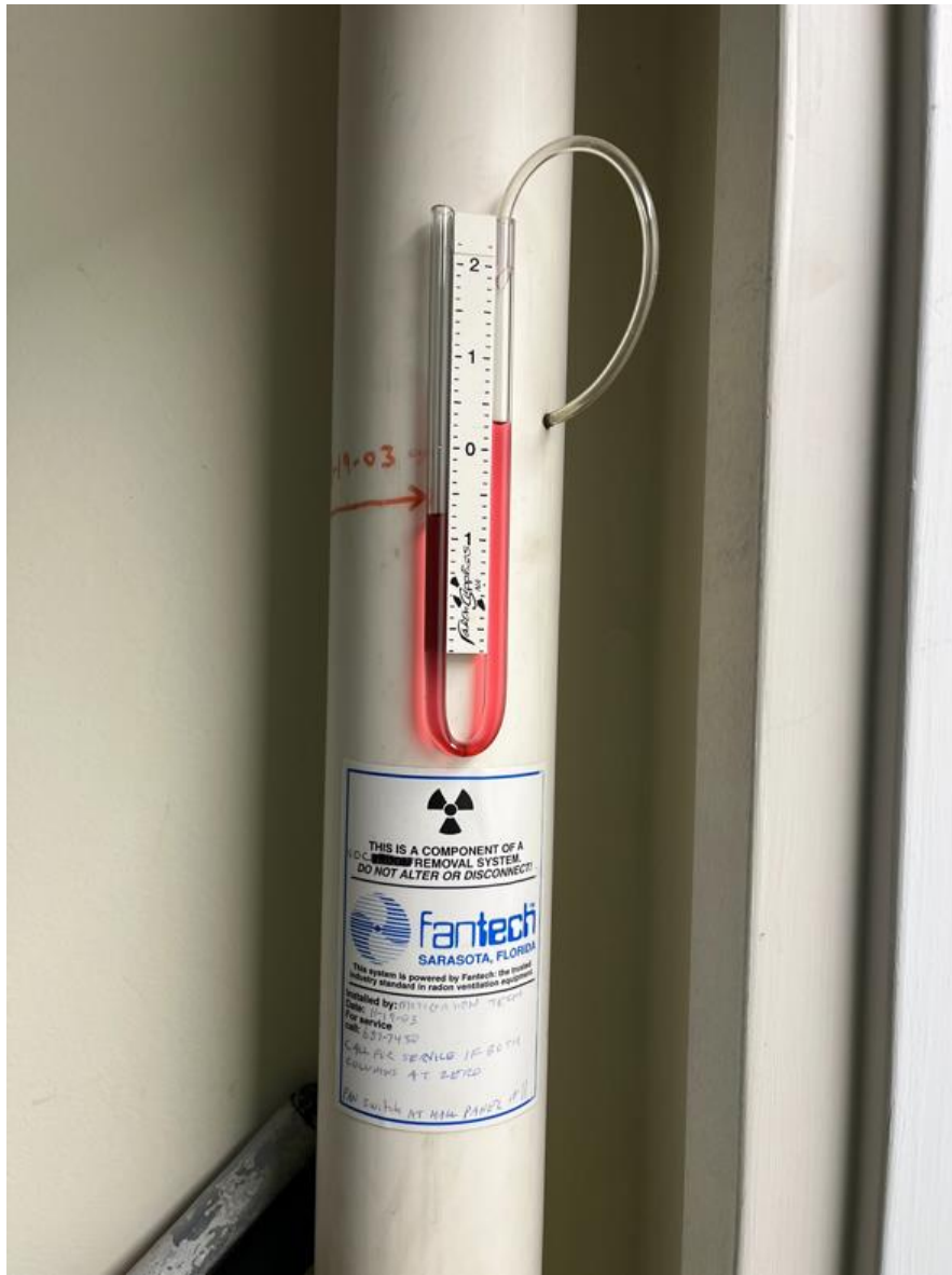
Sub-Slab Depressurization System October 30, 2022
