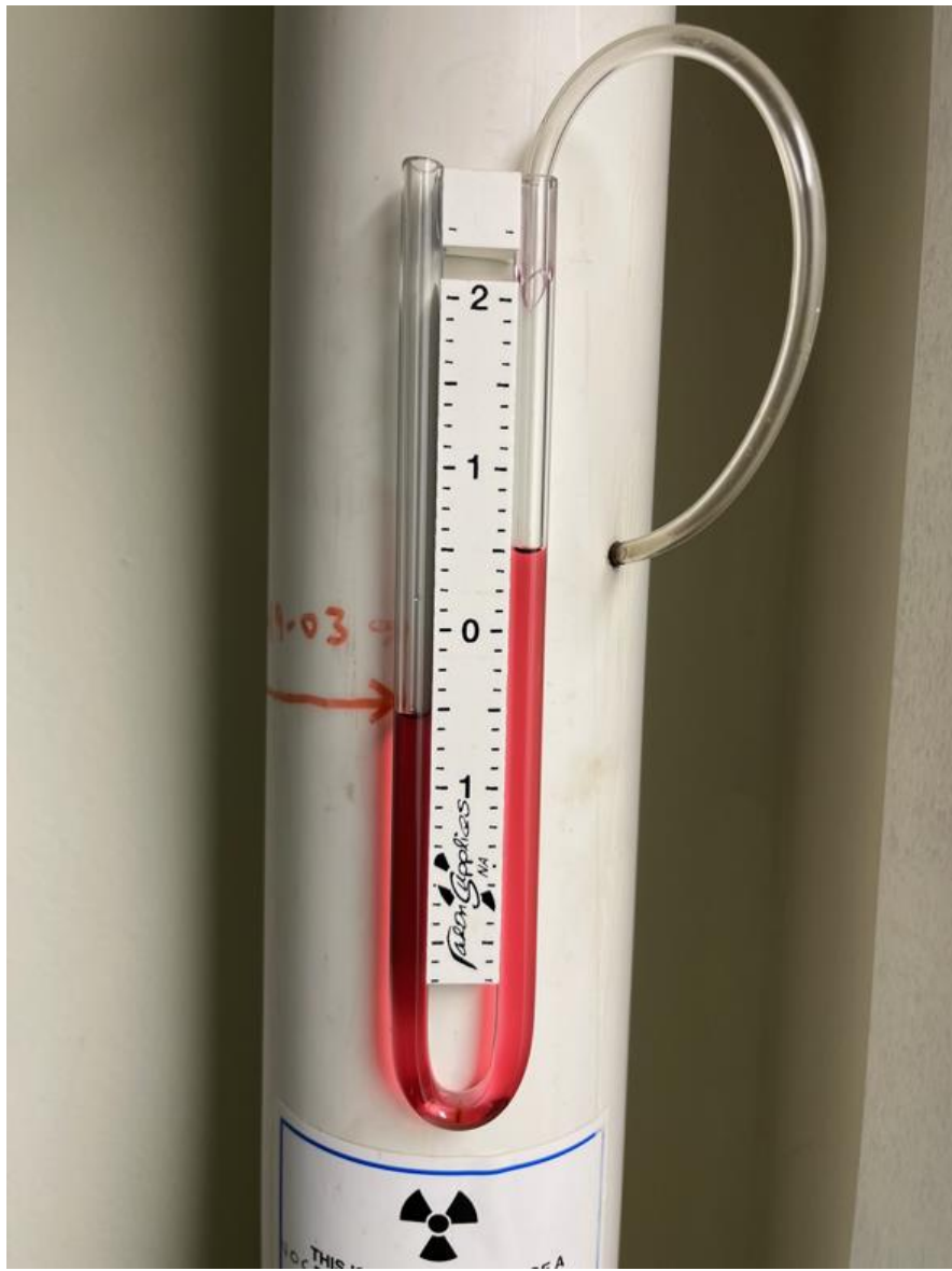
Sub-Slab Depressurization System April 12, 2024
