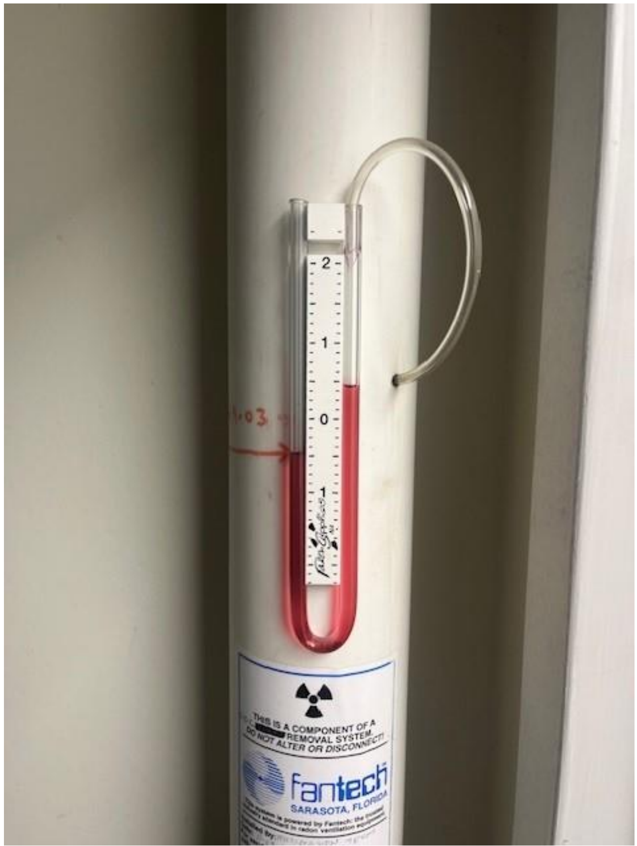
Sub-Slab Depressurization System November 27, 2024
