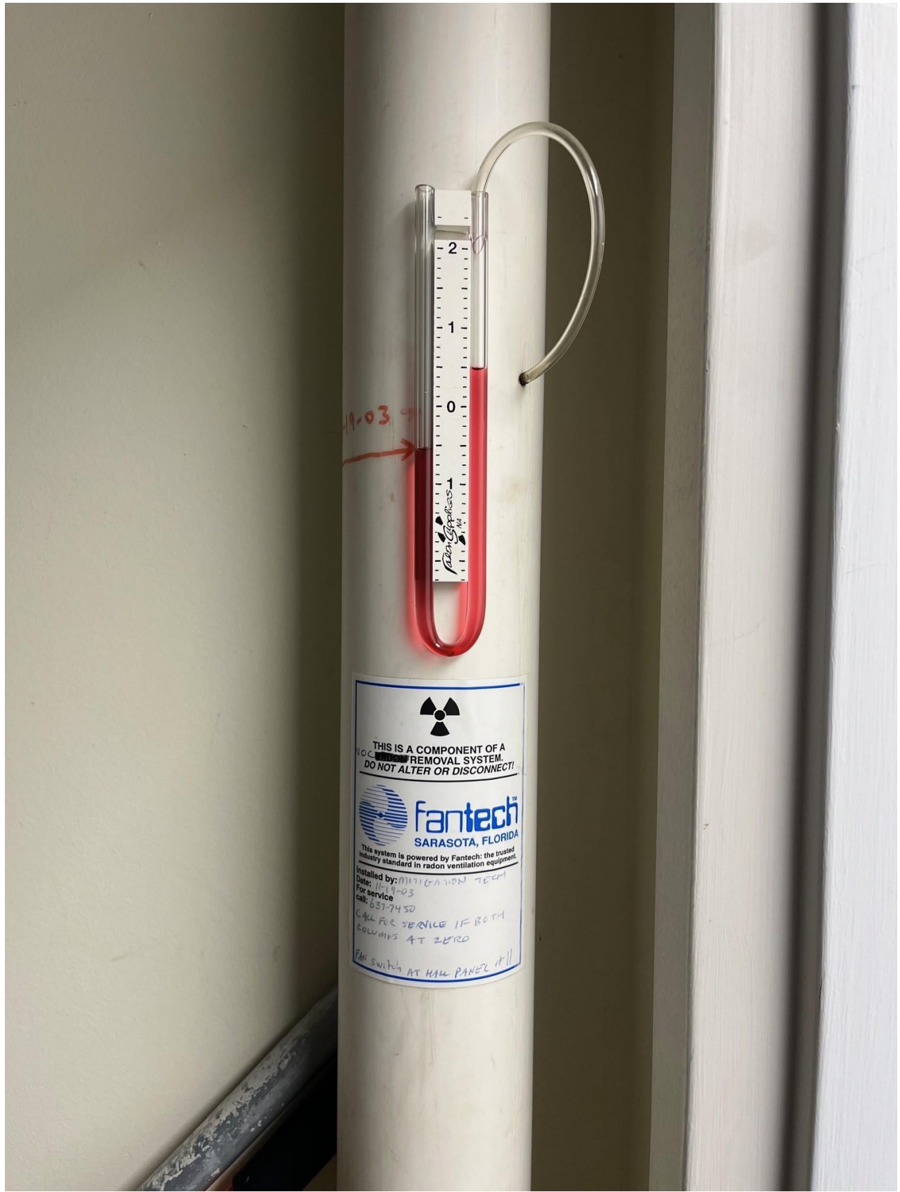
Sub-Slab Depressurization System April 22, 2025
