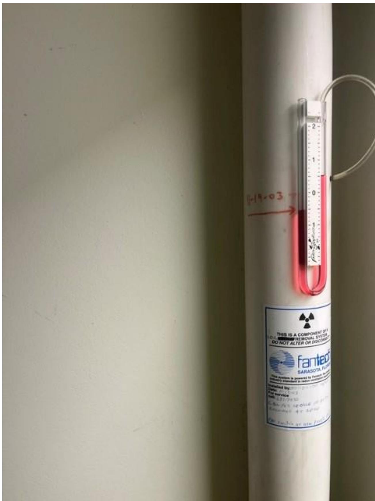
Sub-Slab Depressurization System March 10, 2026
