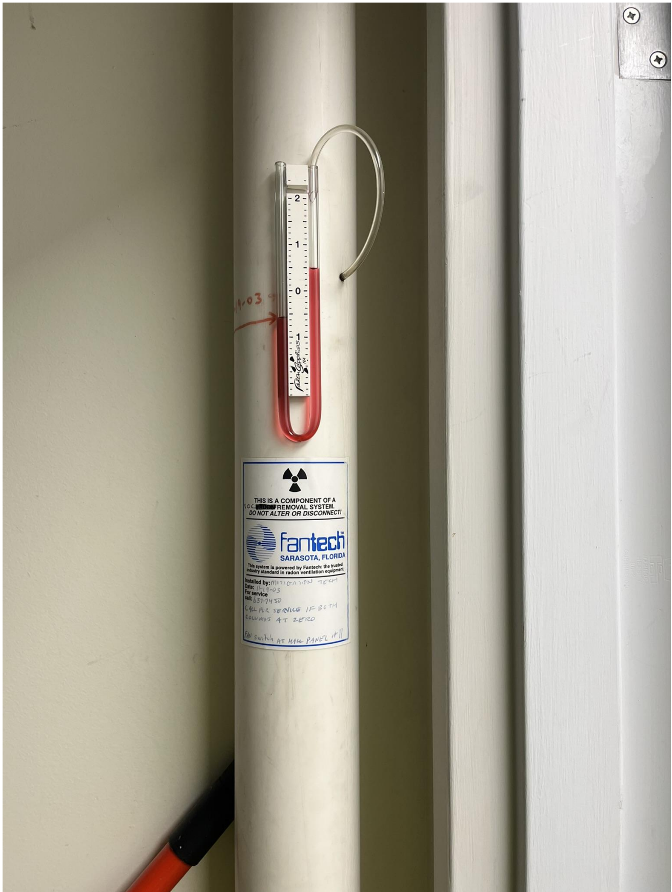
Sub-Slab Depressurization System August 8, 2025
