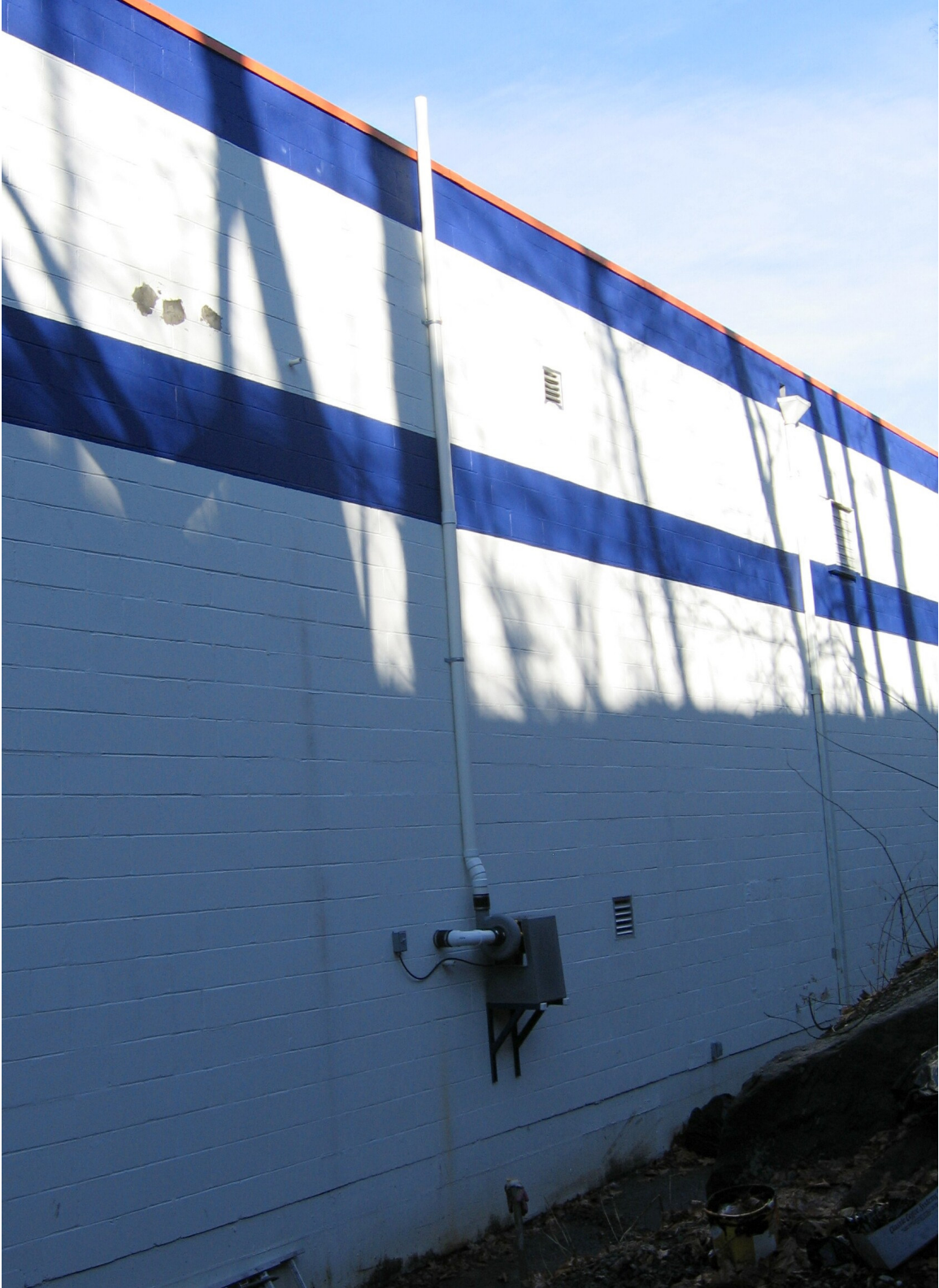
Exhaust Fan 3, Building 4
