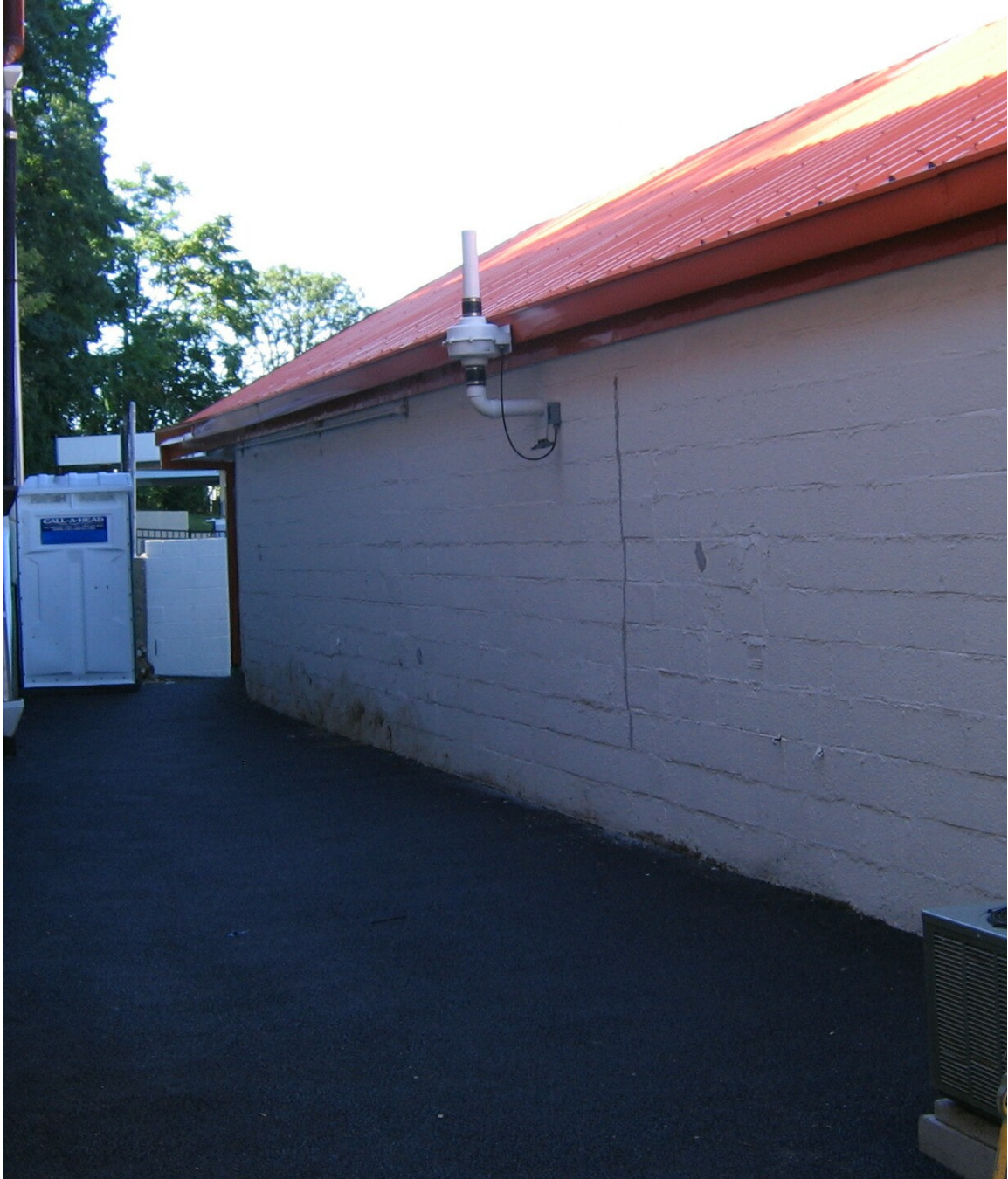
Exhaust Fan 6, Building 9
