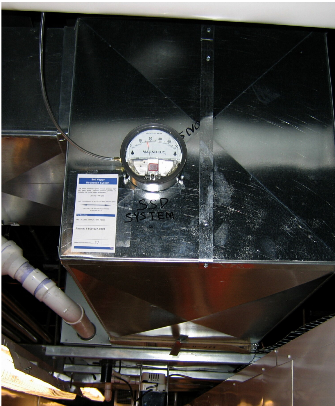
Magnehelic type Manometer Building 1 system (Note pressure reading: 17)
