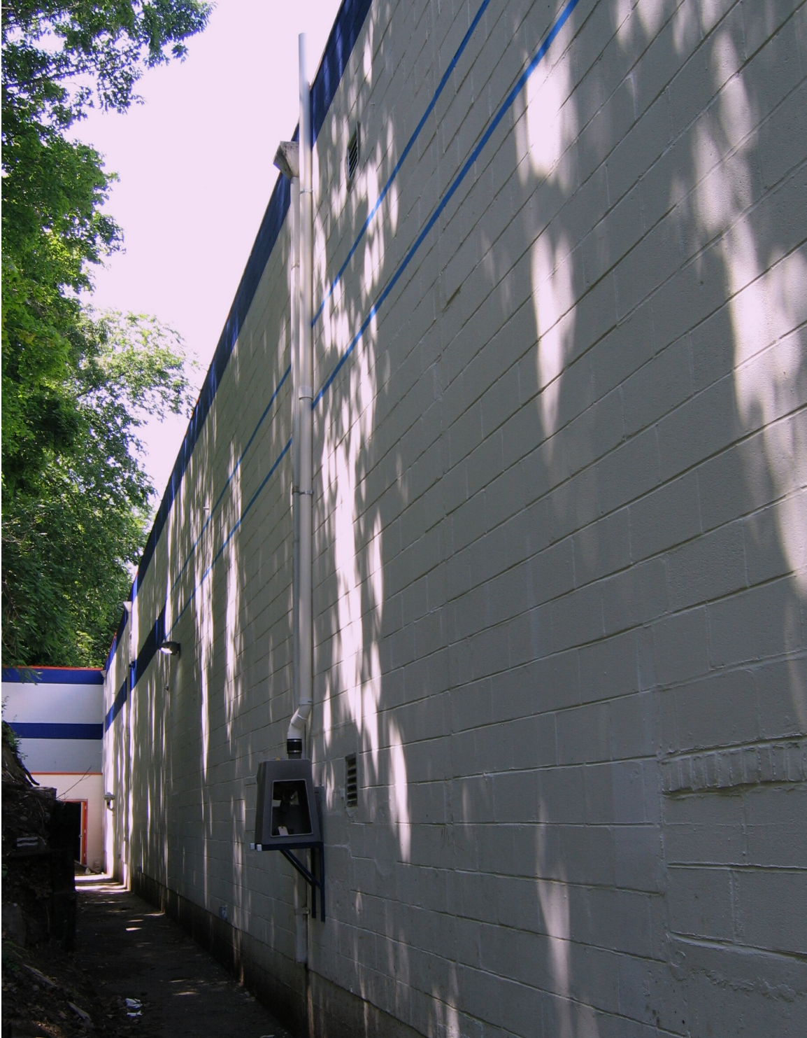
Exhaust Fan 2, Building 4
