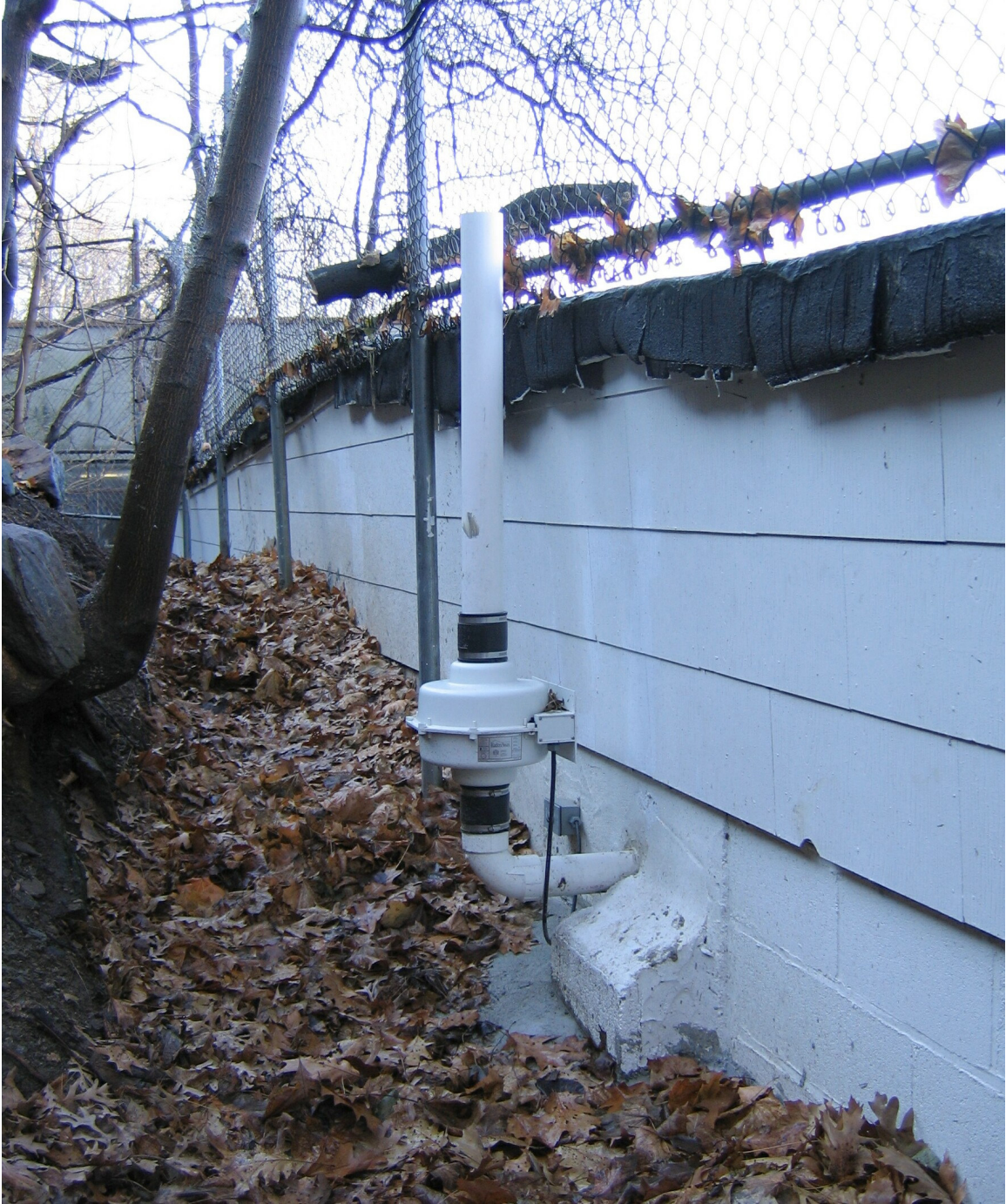
Exhaust Fan 4, Building 6
