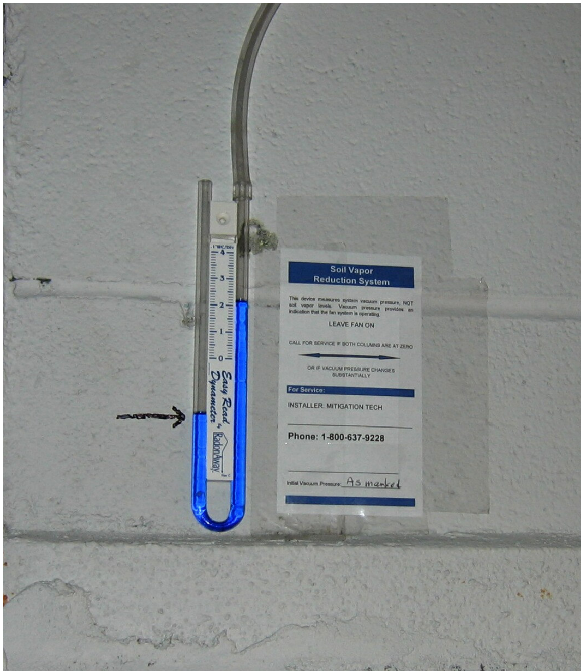
U-tube type Manometer, Building 4, system 2 Type used on systems 2, 3, 4, 5 & 6
