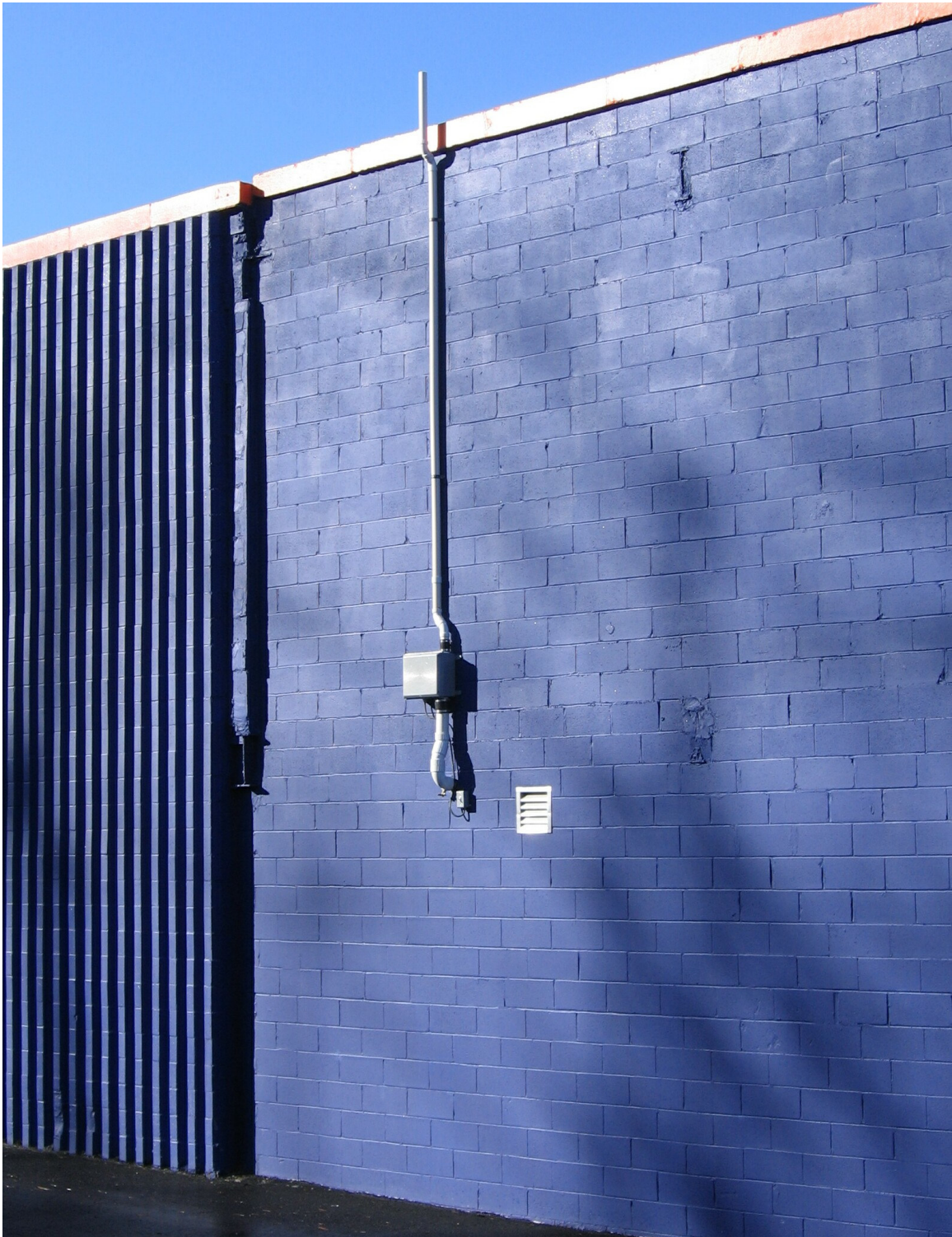
Exhaust Fan 1, Building 1
