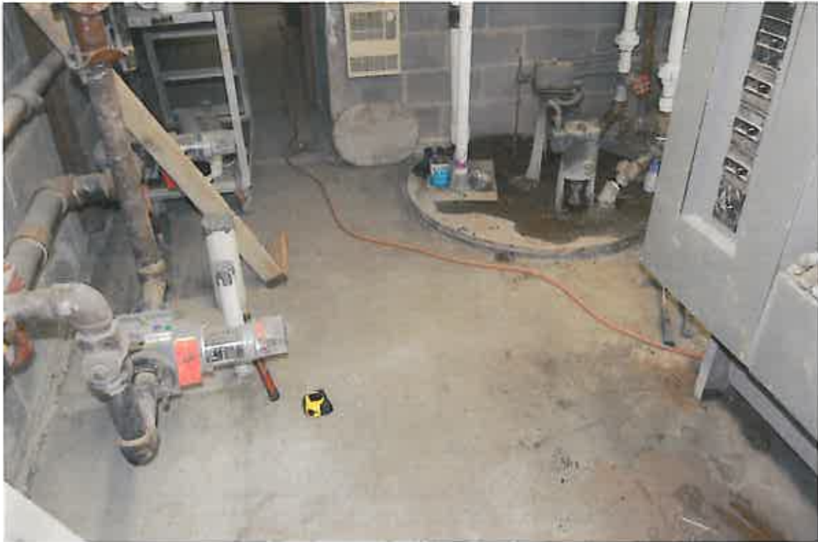
EQUIPMENT ROOM RESTORED
