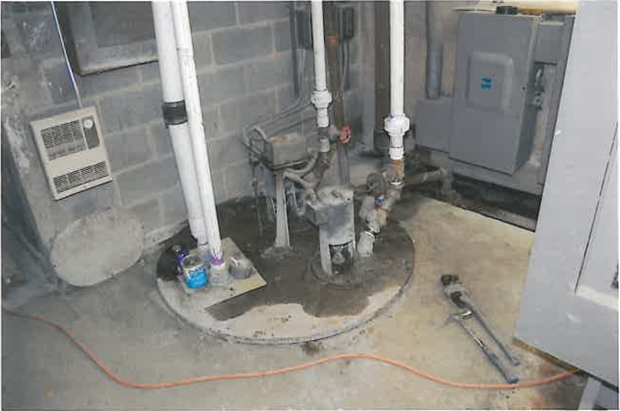
LARGE SUMP PIT WITH NEW PLUMBING
