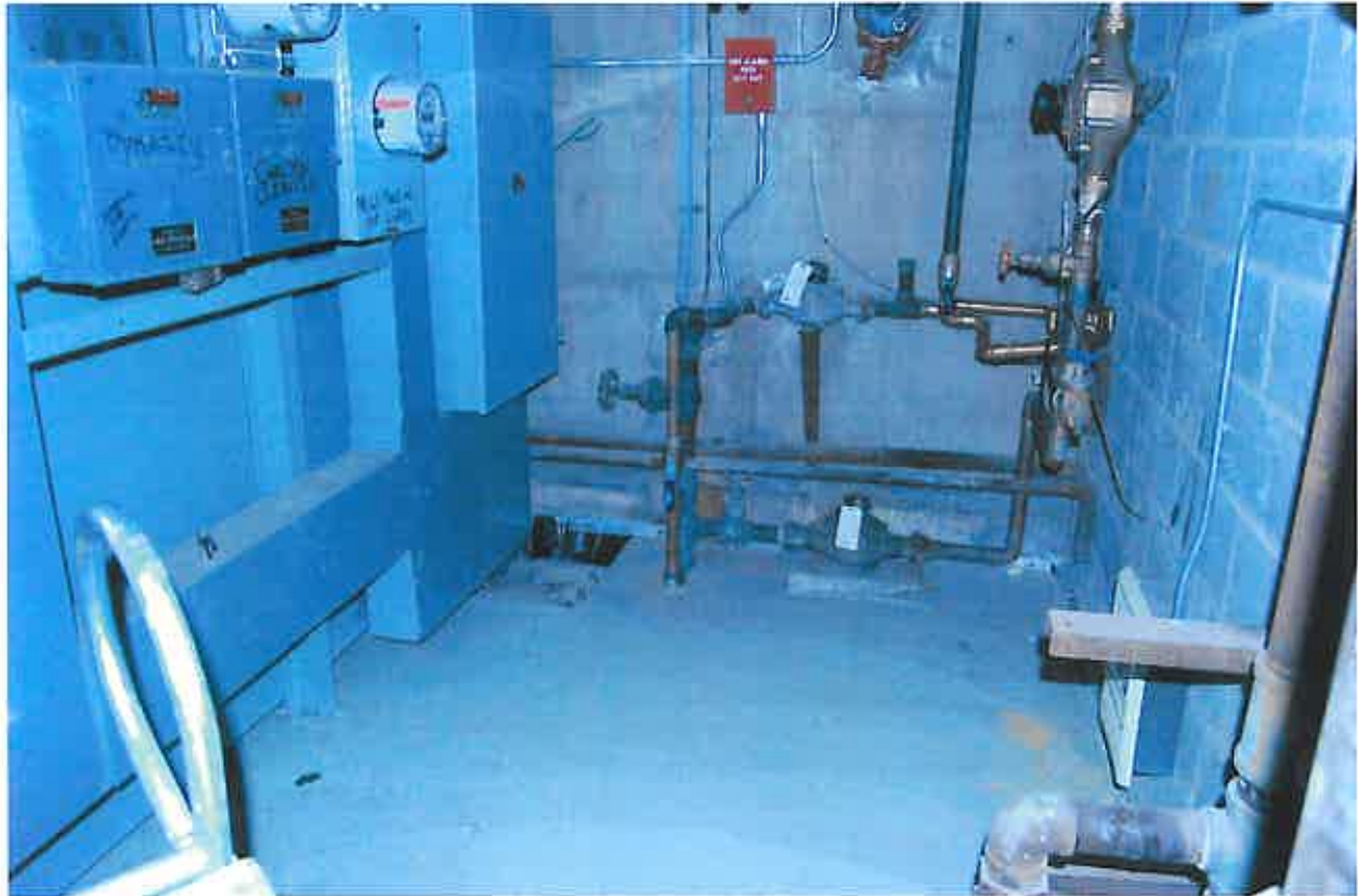
EQUIPMENT ROOM LOOKING EAST
