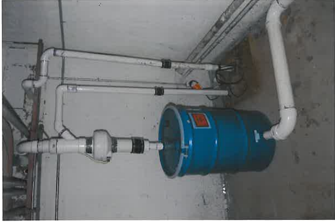
DUCT FAN, VAPOR PHASE CARBON FILTER, SMALL NORTH SUMP PIT
