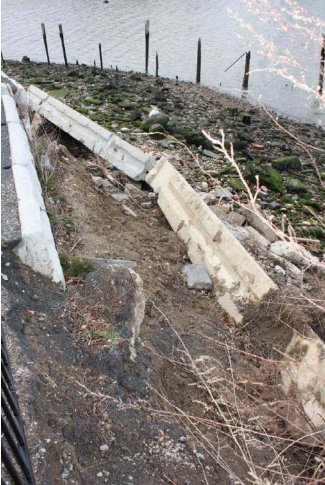
Photograph 9 – Failure of the slope due to wave action and erosion caused failure of the Jersey barrier.
