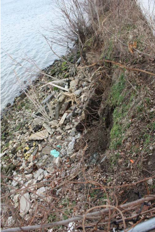
Photograph 12 – Movement of North side of slope requires remediation before the failure extend back to the homes.
