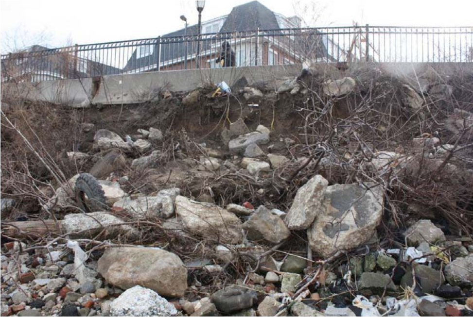
Photograph 3 – Addition of rip rap alone will not secure the Jersey barrier nor prevent future movement.
