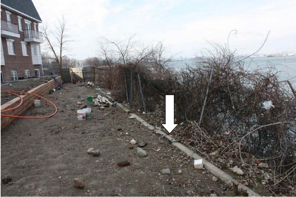
Photograph 10 – Jersey barrier being used as retaining wall is beginning to become undermined and shift seaward.
