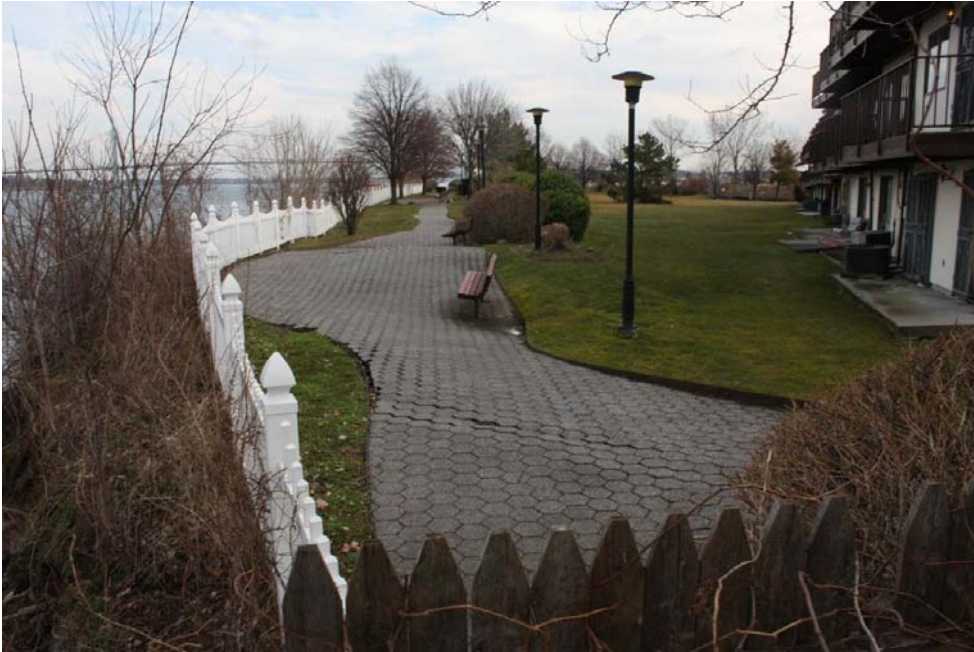
Photograph 13 – Movement of walkway on property to the East indicates movement of the slope.
