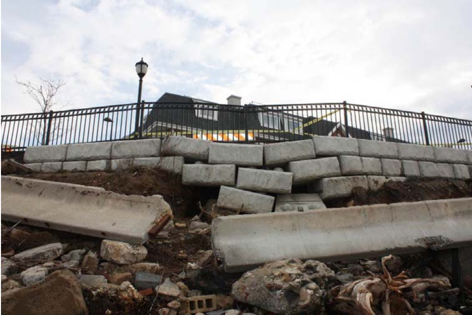
Photograph 4– Failure of the slope due to wave action and erosion caused failure of the Jersey barrier and subsequent movement of the retaining wall.
