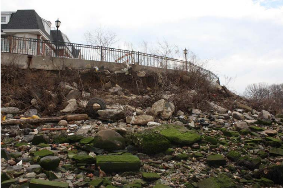
Photograph 7 – Erosion of soil will cause Jersey barrier to collapse in the near future.
