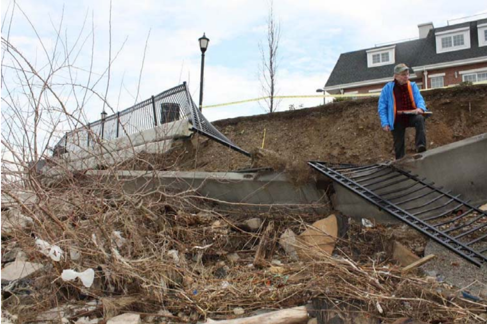
Photograph 8– Failure of the slope due to wave action and erosion caused failure of the Jersey barrier.
