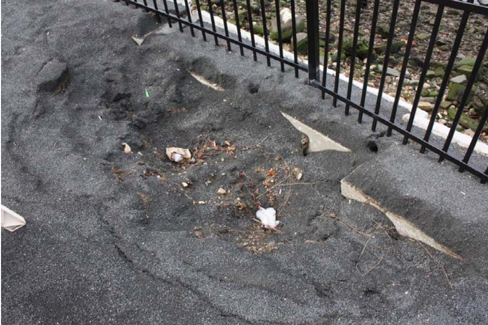
Photograph 2 – Sinkhole forming in walking path where soil was washed out below.
