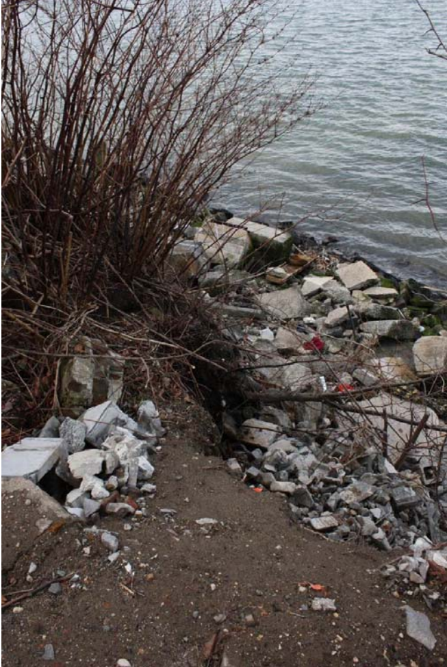
Photograph 11 – Washout of North side slope will lead to failure of seawall rip rap and leave townhouses exposed to the East River.
