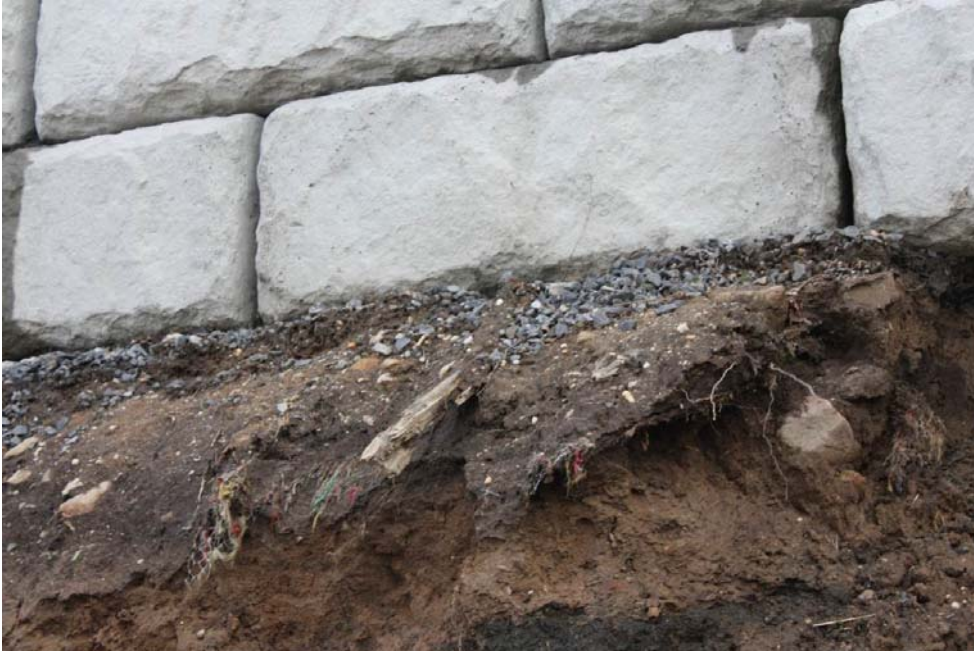
Photograph 6 – Soil erosion due to wave action responsible for the collapse. Gravel setting bed is being undermined by erosion of soil.
