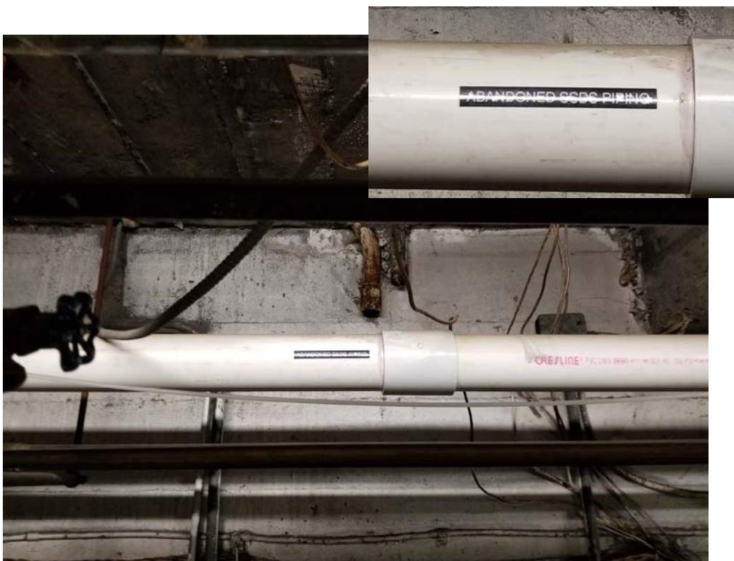
PHOTO 5: LABELED CAPPED LATERAL PIPING REMAINING IN PLACE
