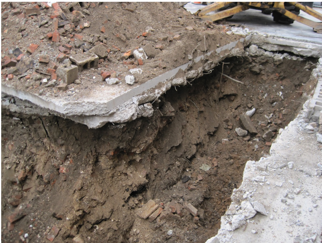
Photo 6: View of corner of test pit TPD-3,.
