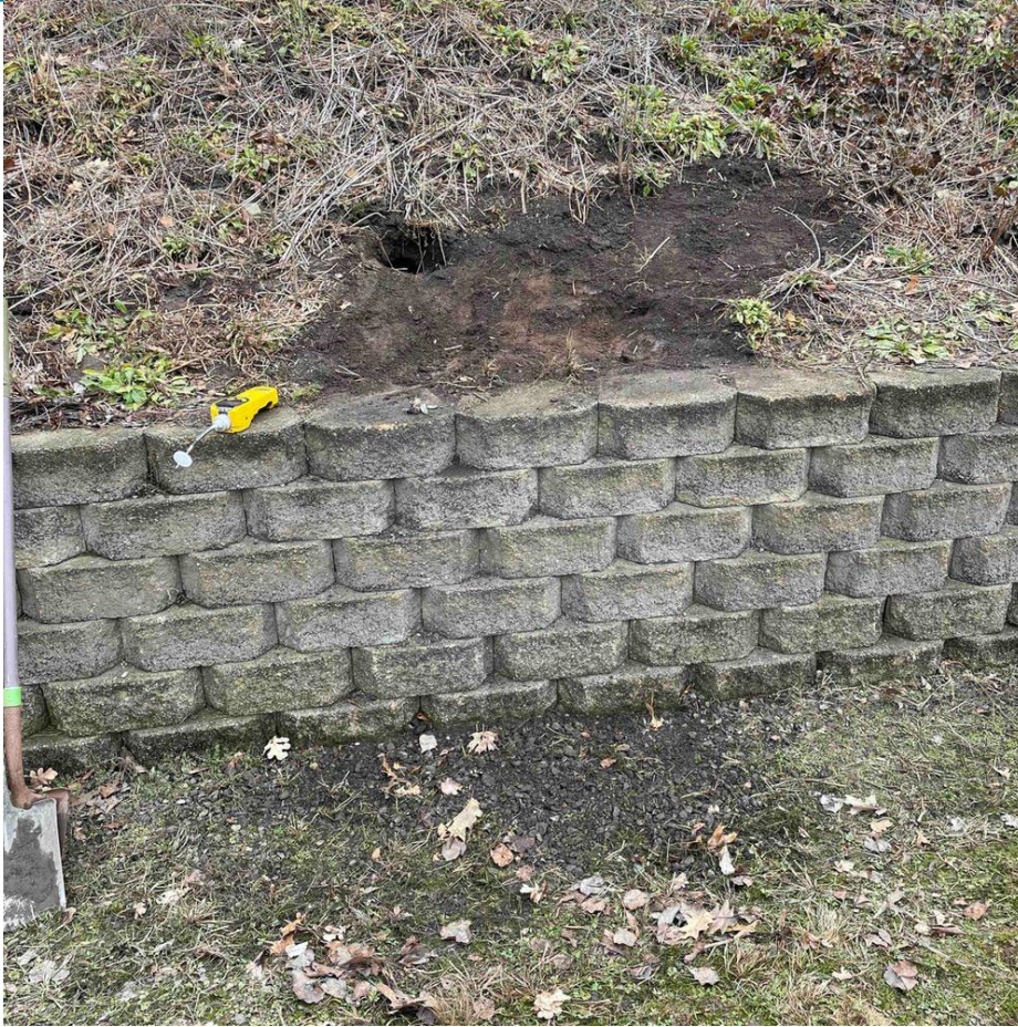
Photo 2: Material removal at animal burrow. Photograph taken 2-17-2023.
