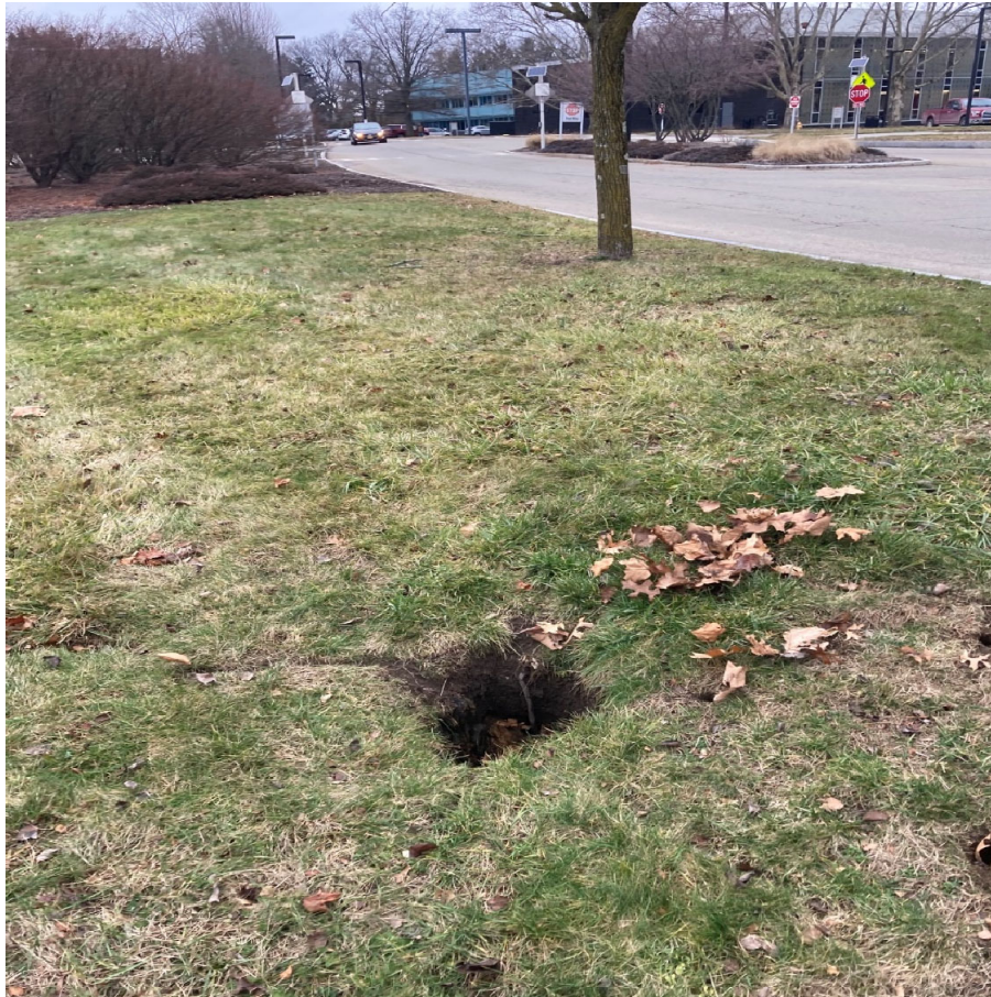
Photo 7: Surficial ground depression in north area of property.
