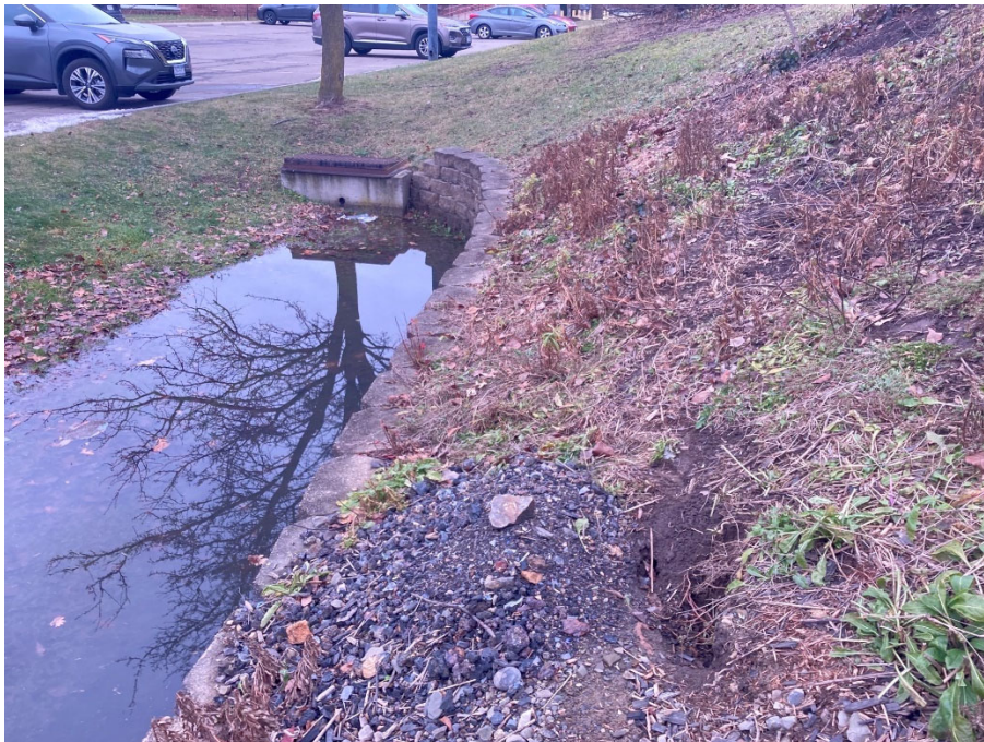
Photo 6: Cover breach in southeast corner of property caused by wildlife.
