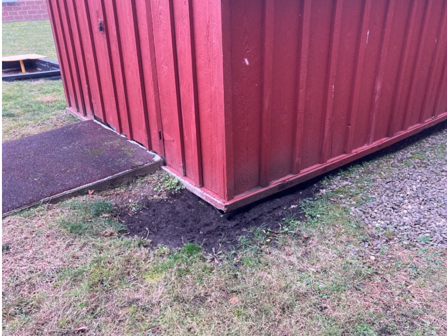
Photo 5: Surficial ground disturbance around shed caused by installation of wildlife deterrent fencing.
