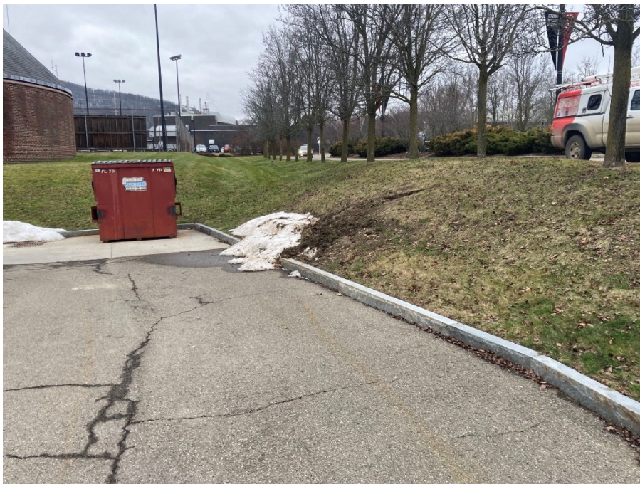
Photo 4: Surficial ground disturbance in north area of property caused by snowplow.
