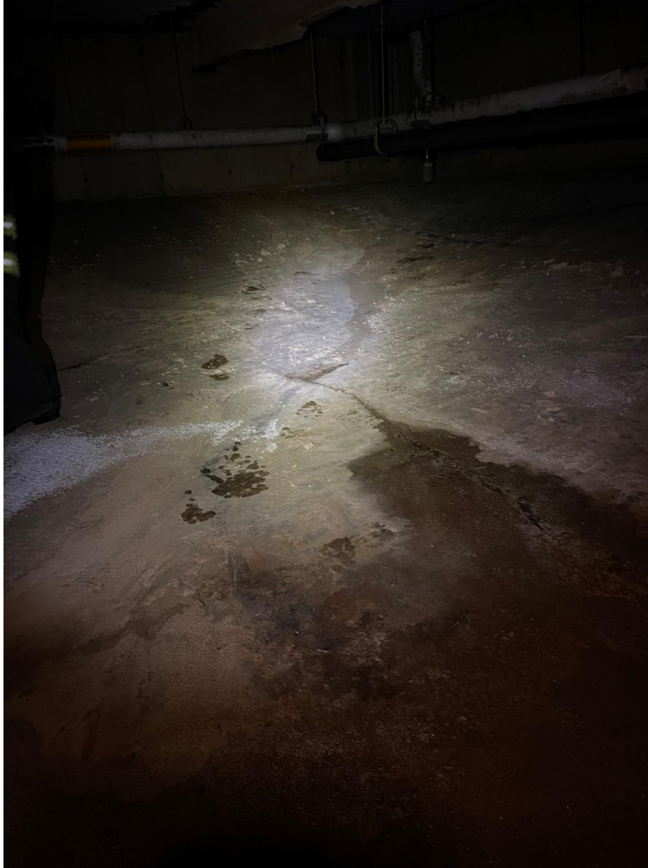
Photograph 6: Corner of floor and sloped wall moving left from manometer. (Note apparent water path down sloped corner. Potential source in sidewall.)
