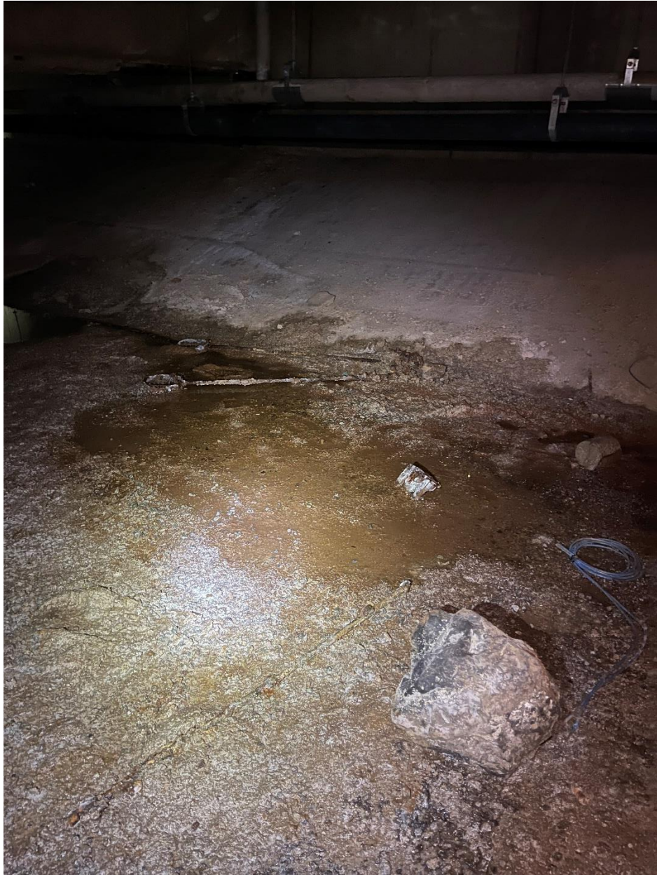
Photograph 5: Typical condition of floor with moisture and debris
