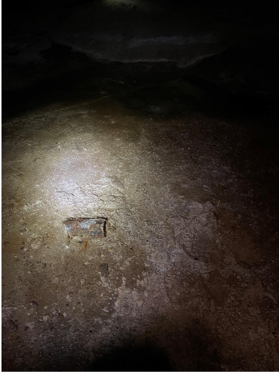
Photograph 9: Debris, typical floor condition.
