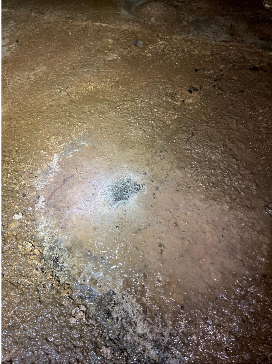
Photograph 13: Water apparently coming from small hole in concrete flooring.
