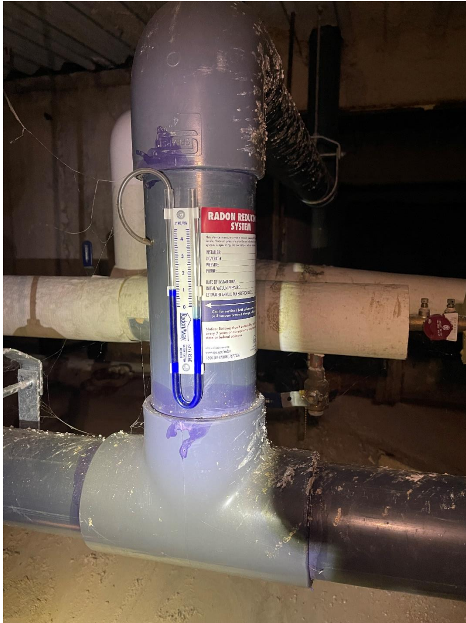
Photograph 3: System manometer (reading 1.0" indicating system is under negative pressure)
