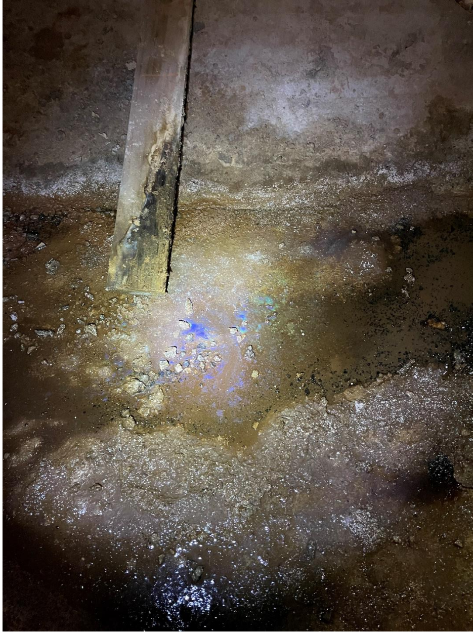
Photograph 11: Sheen present in water.
