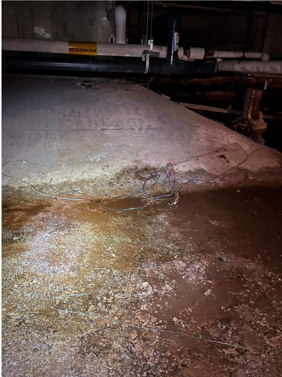
Photograph 4: Floor and sloped wall under manometer (Note debris is accumulated dust, sediment and spalled concrete)
