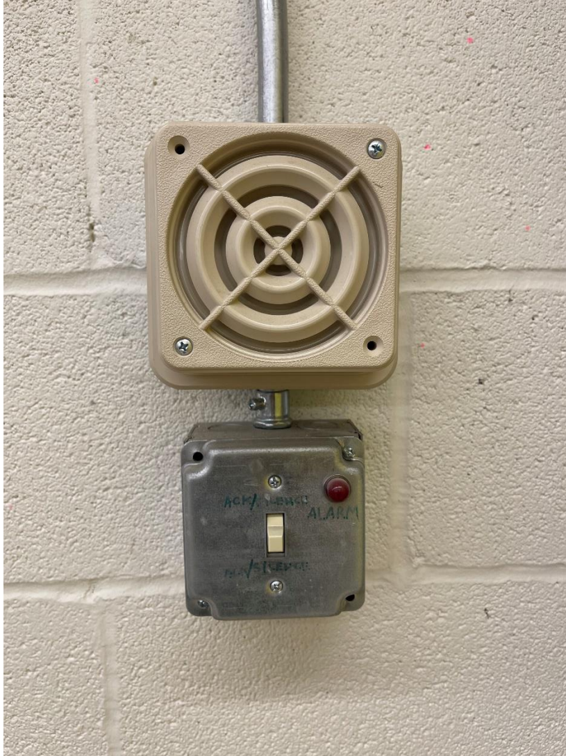
Photograph 1: Alarm for venting system
