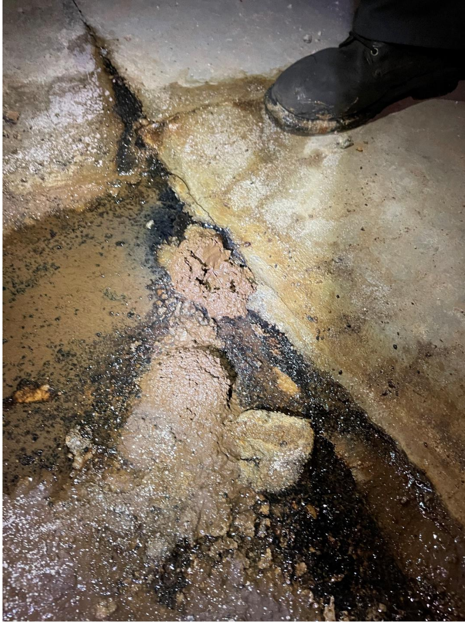
Photograph 12: Bio-mass present near joint in concrete slab floor at sloped wall.
