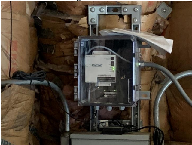
SSDS Alarm System in Treatment Shed
