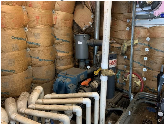
SSDS Blower and Legs in Treatment Shed
