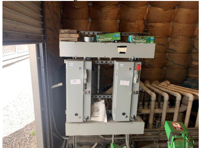
SSDS Blower Electric Panel
