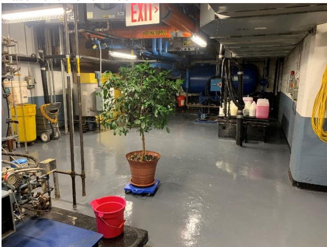
Basement Boiler Room
