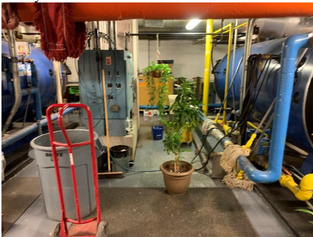
Basement Boiler Room
