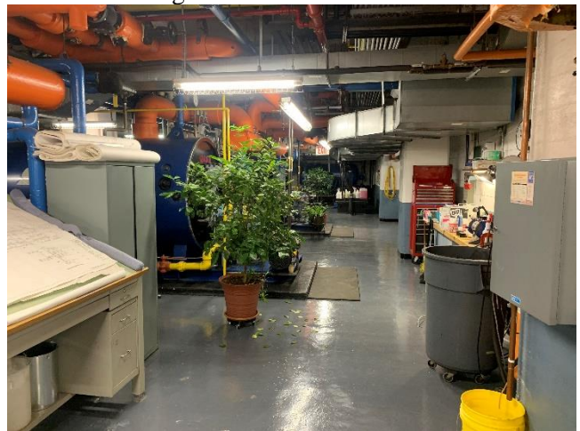
Basement Boiler Room
