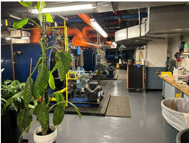
Basement Boiler Room
