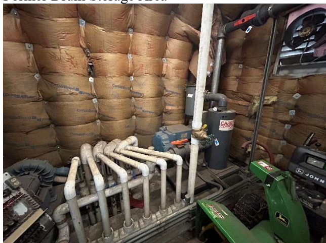
SSDS Blower and Legs in Treatment Shed
