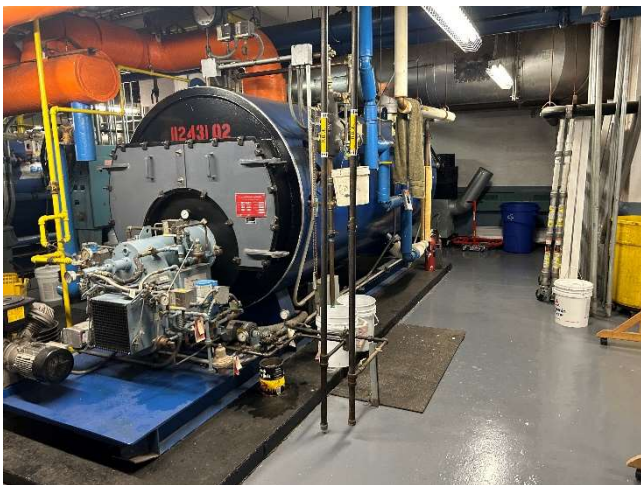
Basement Boiler Room
