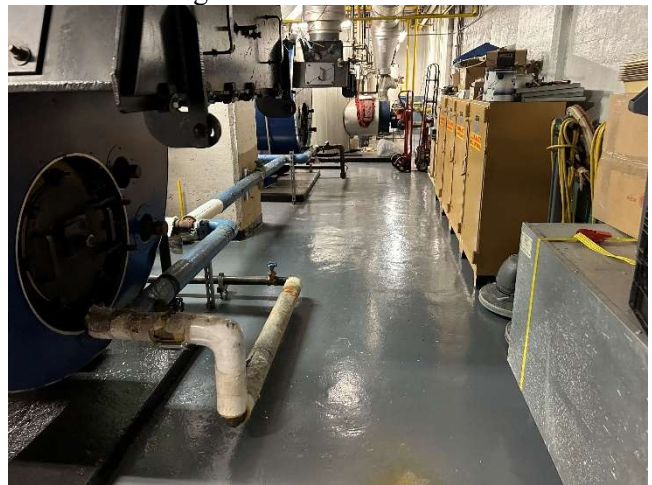
Basement Boiler Room
