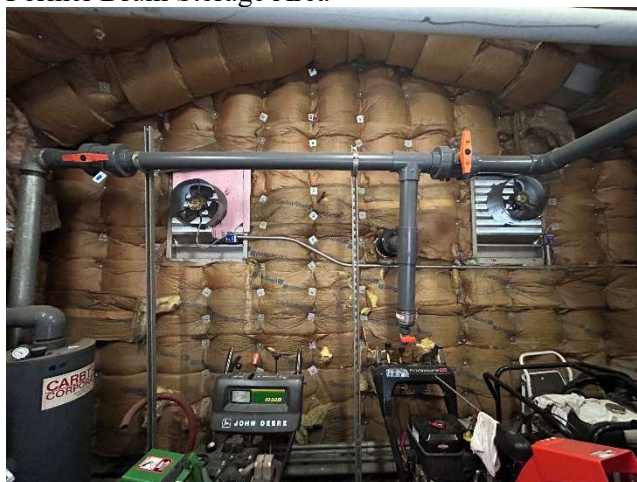
SSDS Blower Electric Panel
