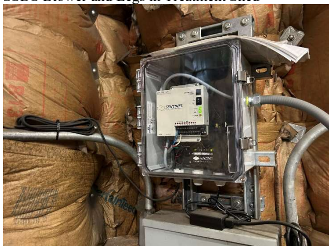
SSDS Alarm System in Treatment Shed
