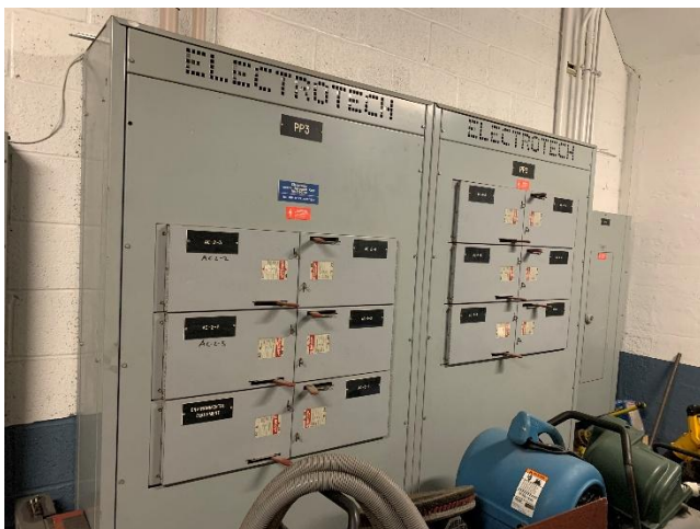
Basement Electrical Room
