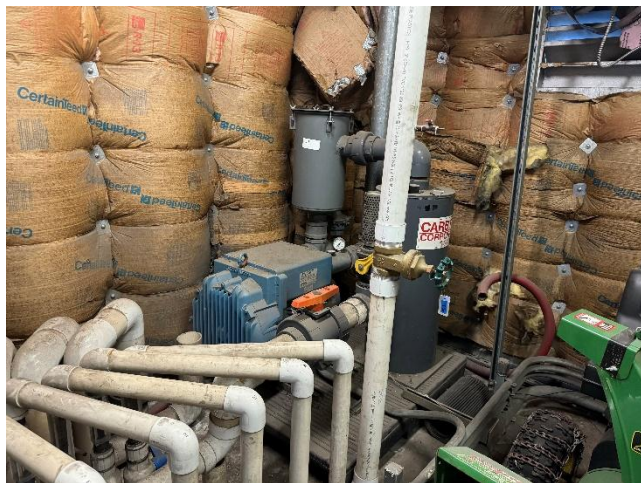
SSDS Blower and Legs in Treatment Shed
