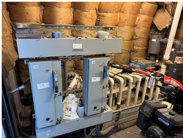
SSDS Blower Electric Panel
