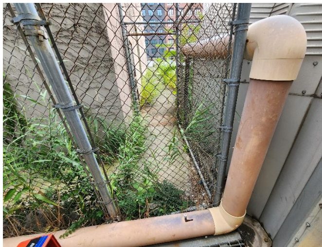
Exterior SSDS exhaust and sampling location
