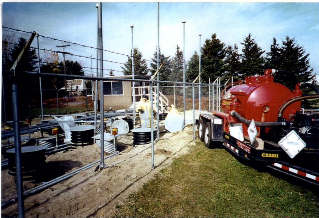
PHOTOGRAPH #3: VACUUM TRAILER
