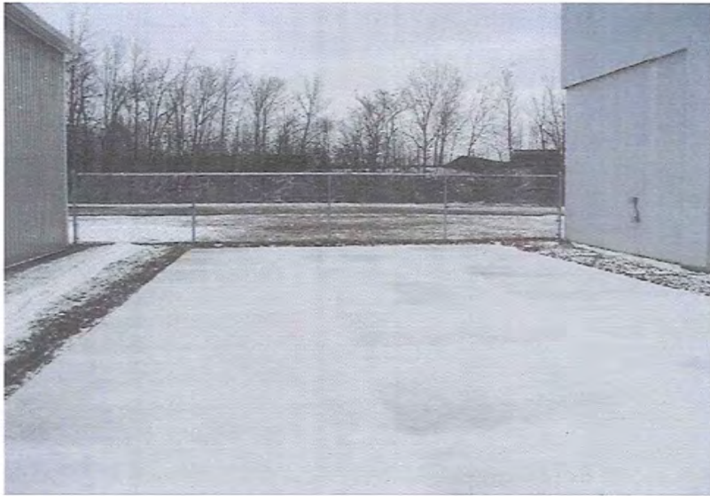
1. New cement pad west side of property between pole barn and building facing east
