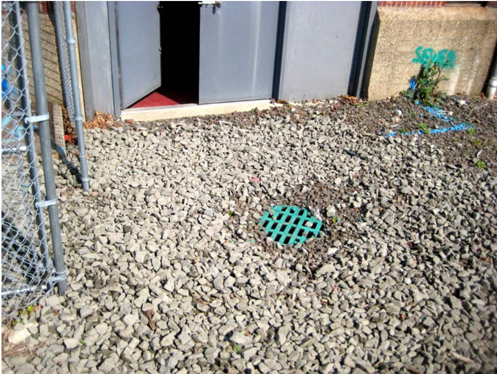
Stone installed in the fenced area south of the swing-out doors on the south side of the substation building.
