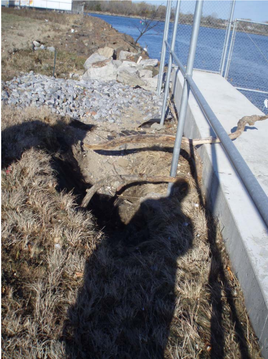
Photograph 2: Erosion observed on the north end of the sea wall (looking north).
