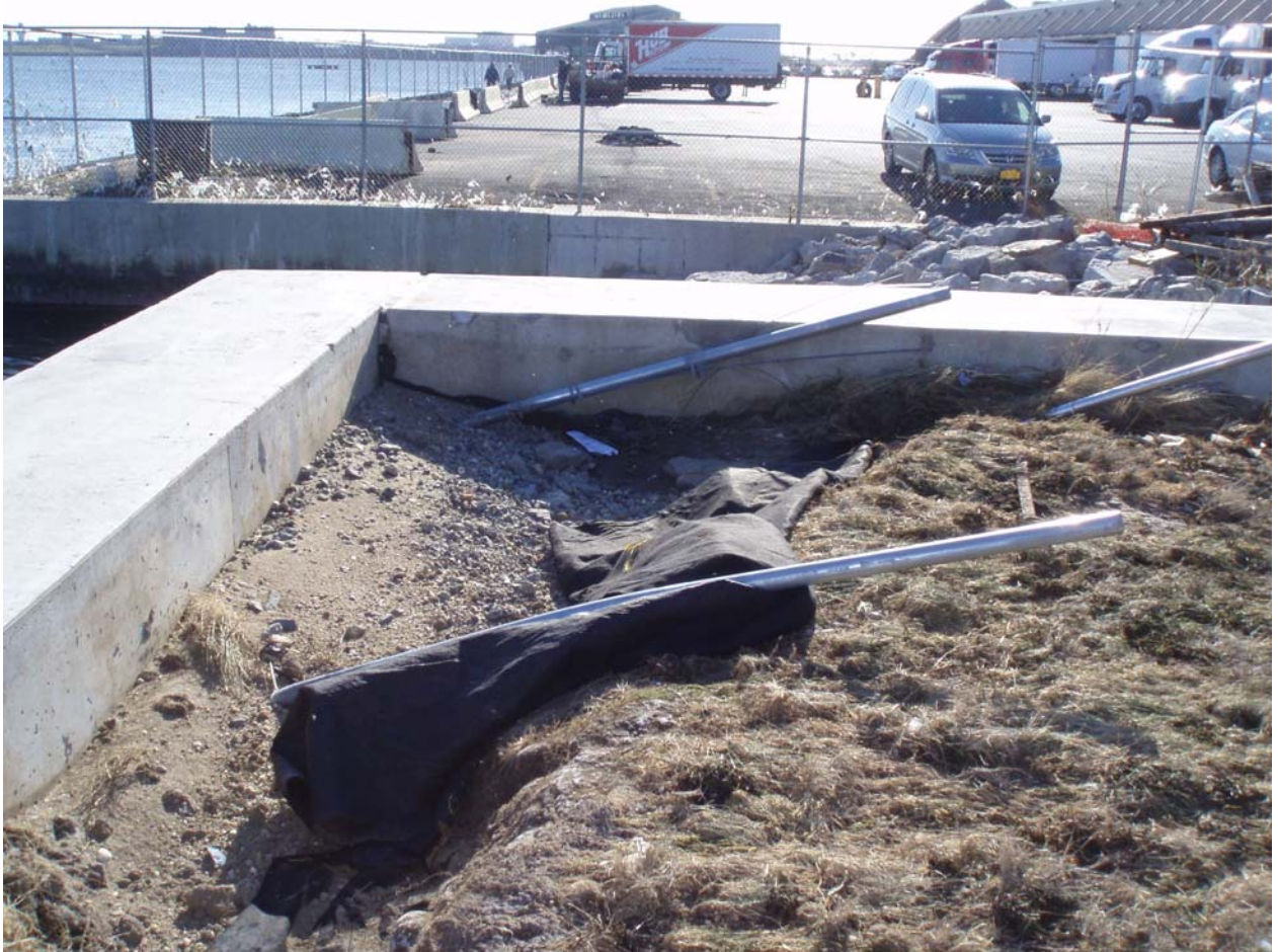
Photograph 3: Erosion observed on the southern end of the sea wall next to Iroquois pipeline (looking south).
