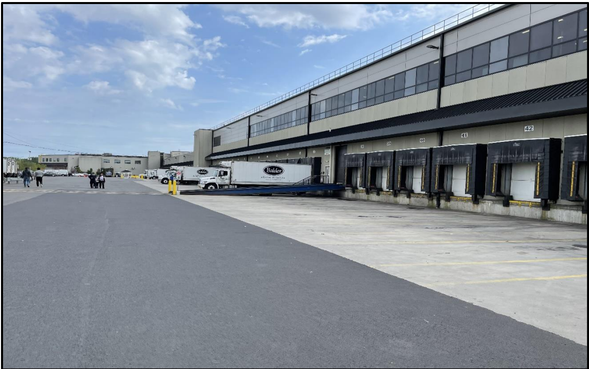
Photo 10: Facing east in the northern portion of the site; asphalt and reinforced concrete slab in truck loading docks in good condition.
