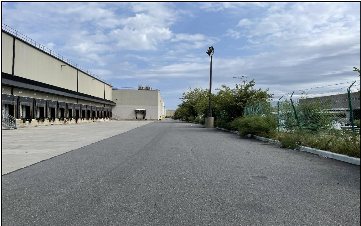
Photo 6: Facing southeast along the southern Site E OU-1 fence line; asphalt and reinforced concrete slab in the southern truck loading dock in good condition.
