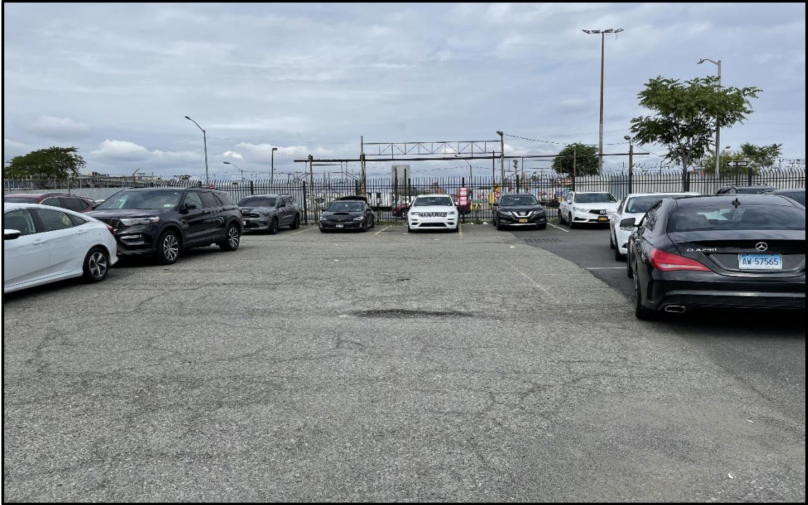
Photo 9: Facing north in the northern portion of the site; pothole observed in the employee parking lot.
