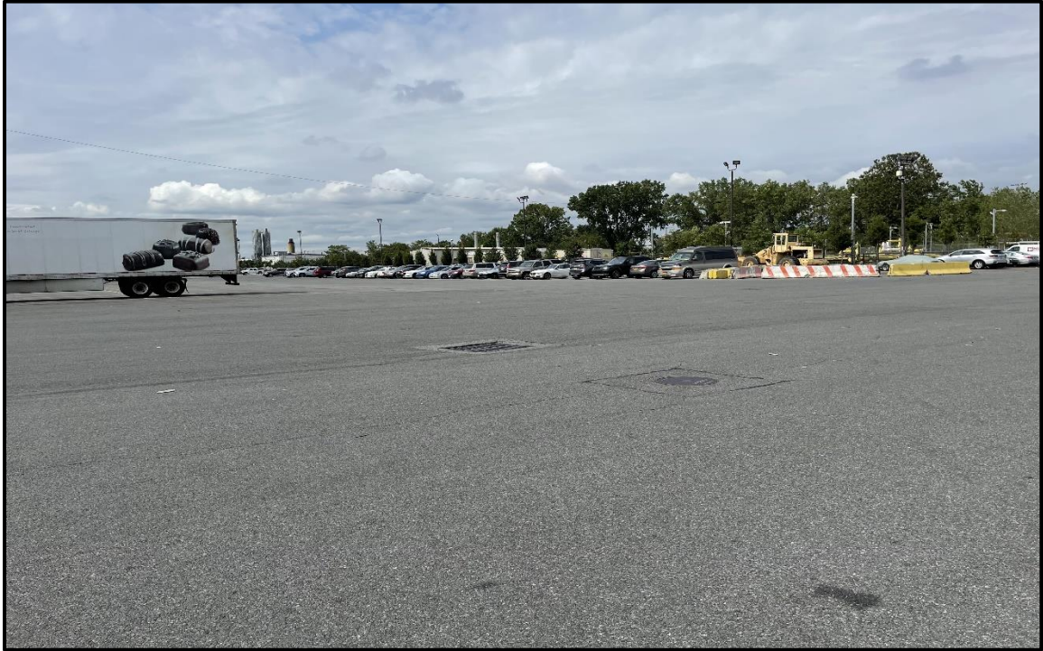
Photo 3: Facing northwest in the western portion of the Site; engineering controls are in place and in good condition adjacent to truck loading docks and truck parking lot.
