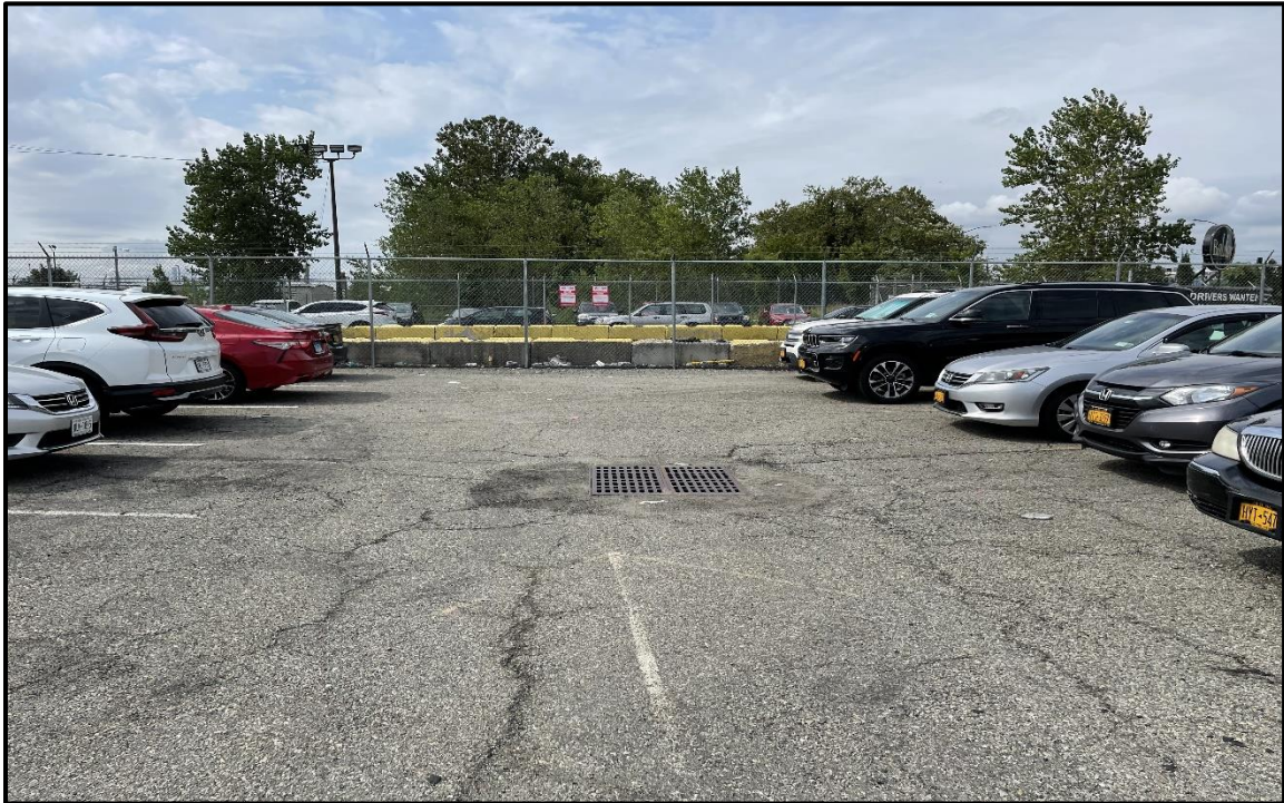
Photo 7: Facing west in the northern portion of the site; general wear shown in the paved parking lot surrounding the storm drain.
