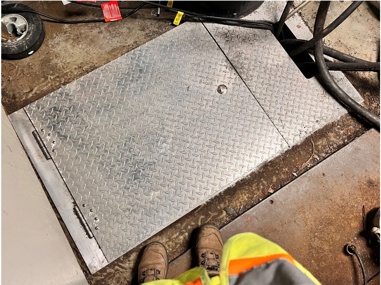
New metal plate covering the sump pit in the SW Pit Room, 10/11/2022.
