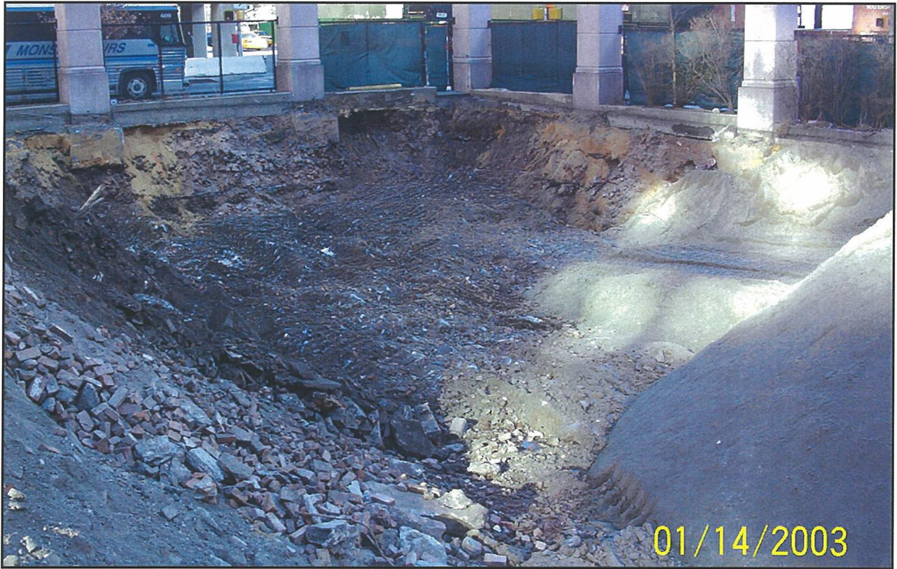
Photo 11. Remedial excavation near northeastern corner of property. Backfilling with imported clean fill in progress.
