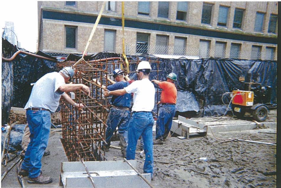
Photo 17. Installation of rebar cage into southeast corner panel of barrier wall prior to placement of concrete.
