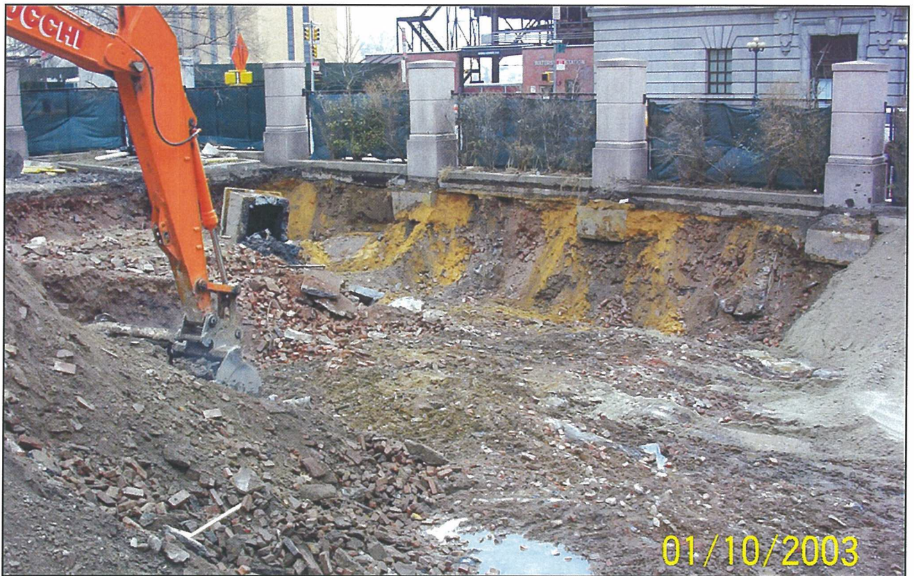
Photo 9. Remedial excavation progress near northeastern corner of property (corner of 40 th St. and First Avenue).
