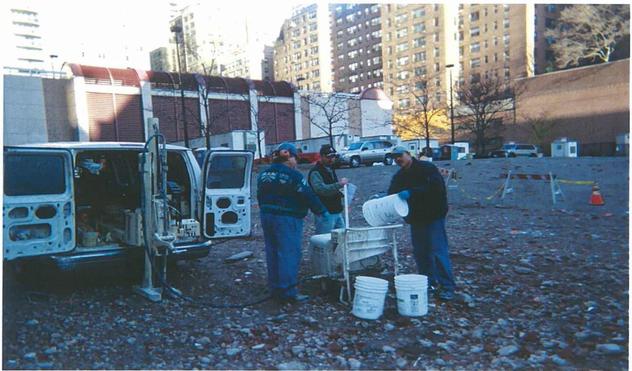
Photo 13. Injection of ORC ® slurry into existing gravel layer above bedrock via Geoprobe ® . ORC ® was applied into 38 injection points in the southeastern corner of the Site between November 18 -19, 2002.
