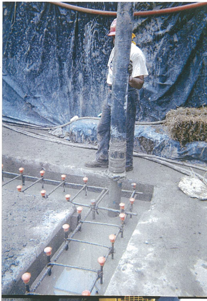
Photo 18. Concrete is pumped into southeast corner panel of barrier wall, displacing slurry.
