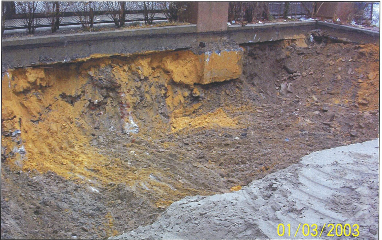
Photo 7. Remedial excavation near the northeastern corner of property at the corner of 40 th St. and First Avenue.
