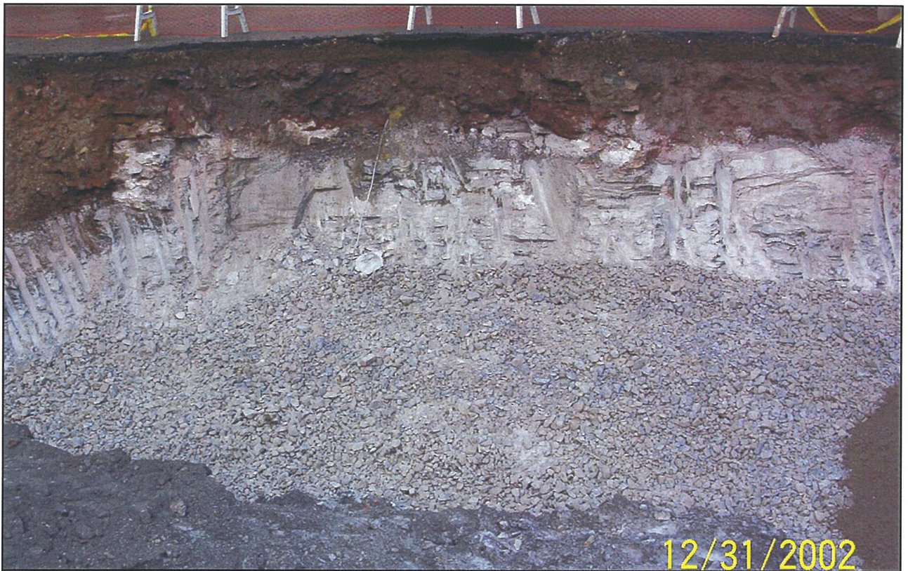
Photo 4. VOC - impacted soil and weathered rock area after a 25% ORC ® solution was applied to the backfilled gravel layer.
