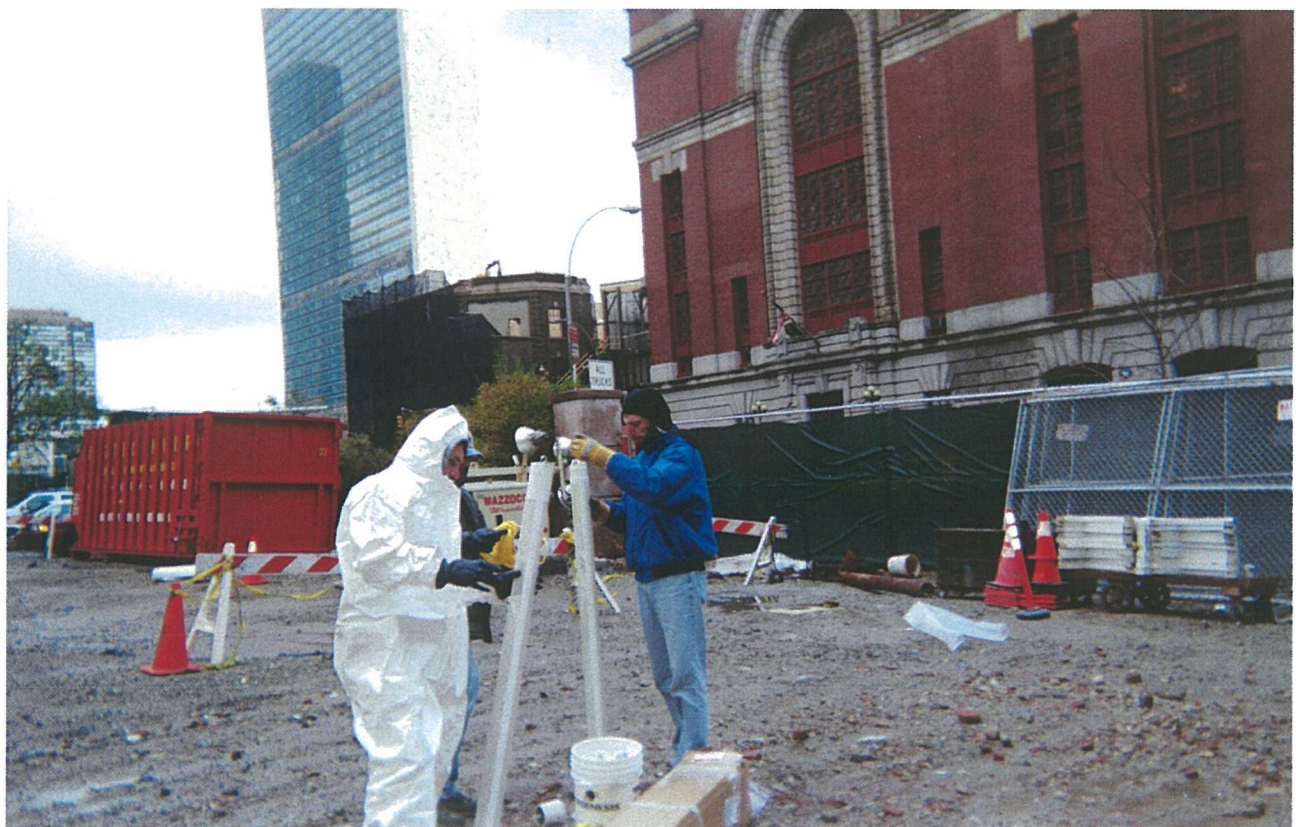
Photo 14. Typical monitoring well installation of permeable ORC ® socks within slotted PVC casing.
