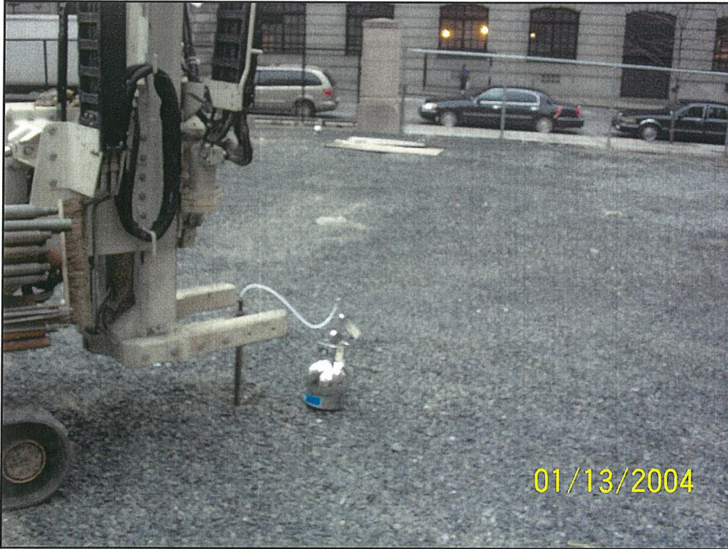
Photo 21. Typical post-remediation soil vapor sample collection at depth of 4' bgs via Geoprobe®. Soil vapor samples were collected at 11 locations, including one ambient background location, on January 13, 2004.
