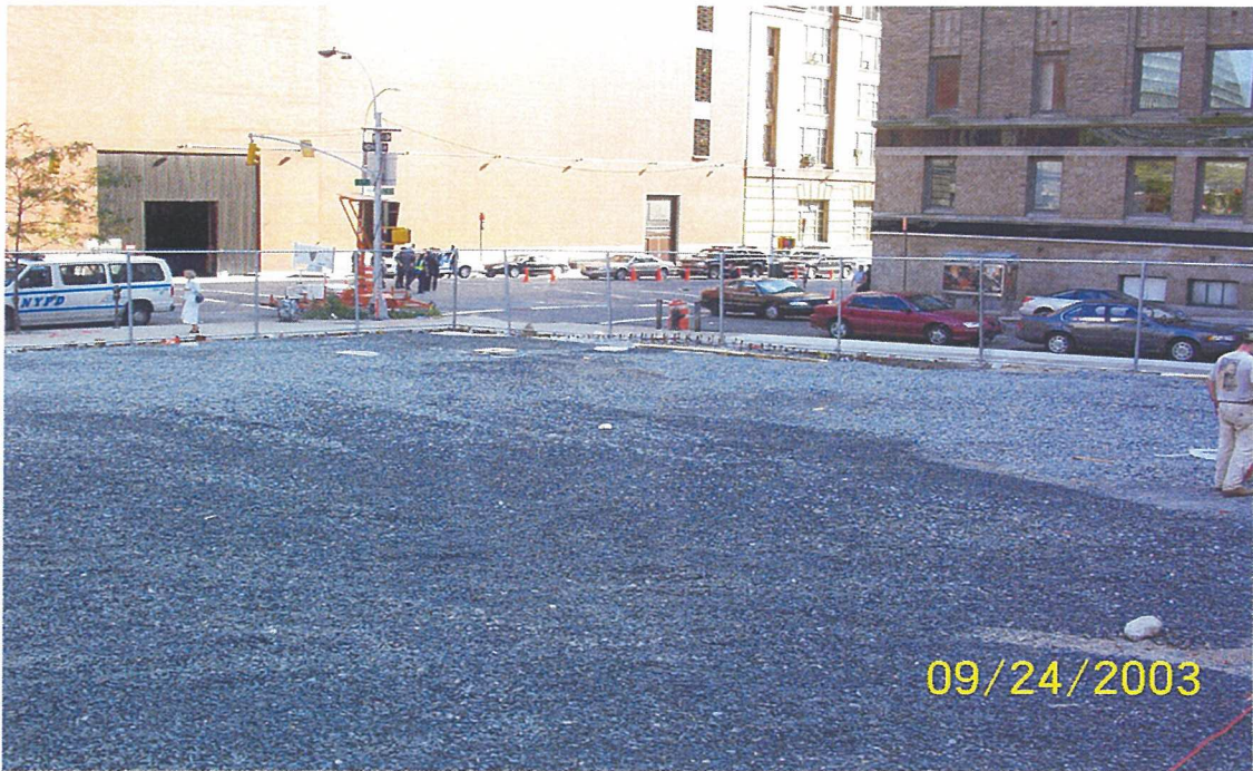
Photo 19. View of southeast corner of Parking Lot Site following completion of remediation and site restoration.
