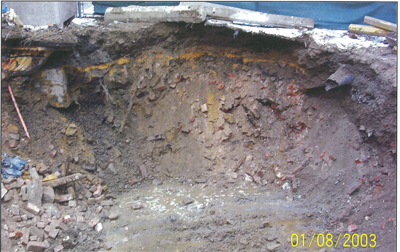
Photo 8. Close up view of fill excavating progress near the eastern extent of remedial excavation along First Avenue.
