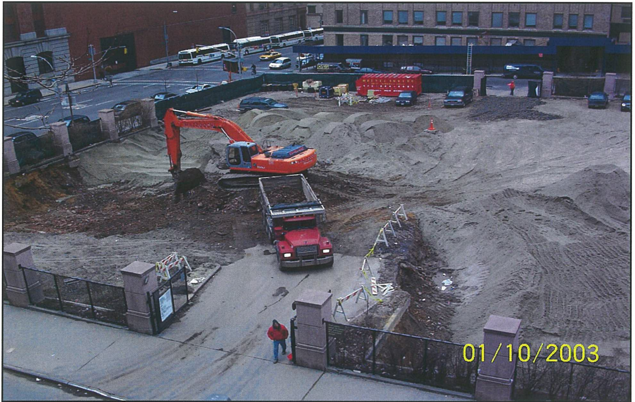
Photo 12. Overhead view of on-going remedial activities at the Parking Lot property. Final excavation of northeast corner of Site being completed, with extensive placement of imported clean fill visible.
