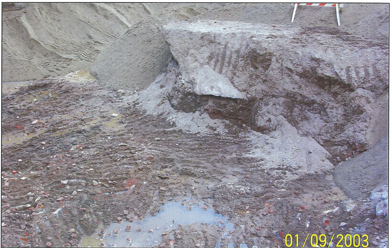
Photo 10. Exposed top of bedrock at eastern extent of remedial excavation prior to it being backfilled with imported clean fill.
