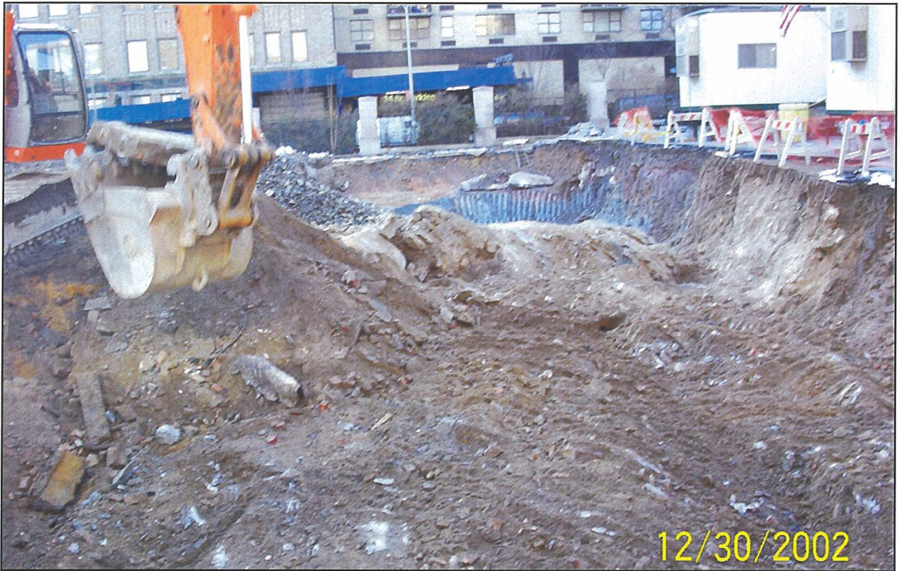
Photo 5. Western extent of remedial excavation looking north to south, spanning across the site from 40 th Street to 39 th Street.
