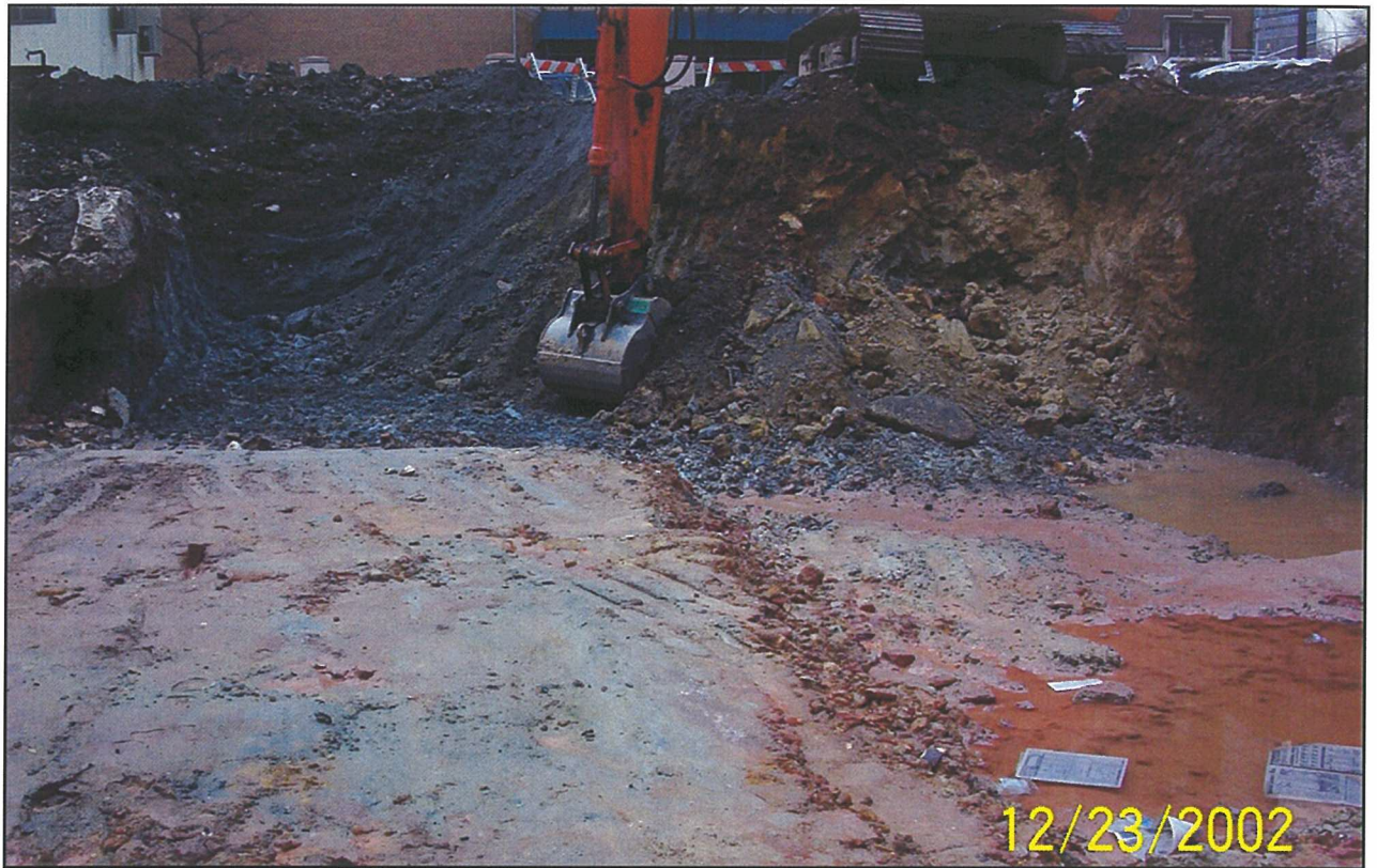
Photo 1. Remedial excavation along Con Edison Utility Easement (western boundary of property). Weathered bedrock is exposed.
