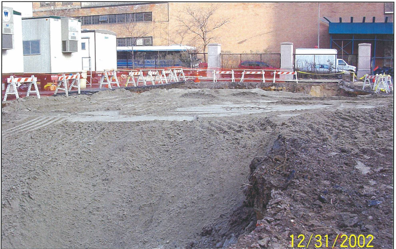
Photo 6. Western extent of remedial excavation along the Con Edison Utility Easement after backfilling with imported clean fill.
