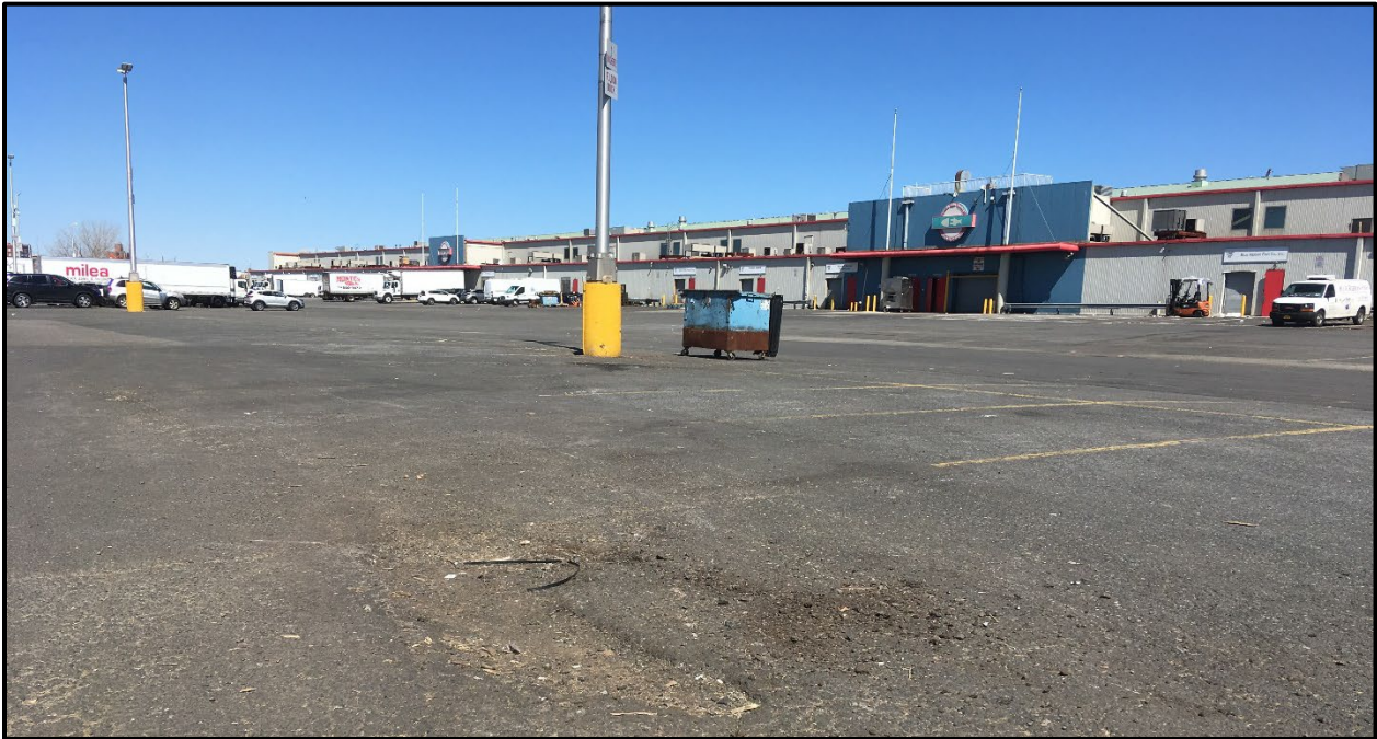
Photo 13: Facing northeast in the western portion of Site; engineering controls are still in place. Normal wear from heavy truck traffic in the form of asphalt cracks and potholes of various sizes are present in the parking lot (March 2019).
