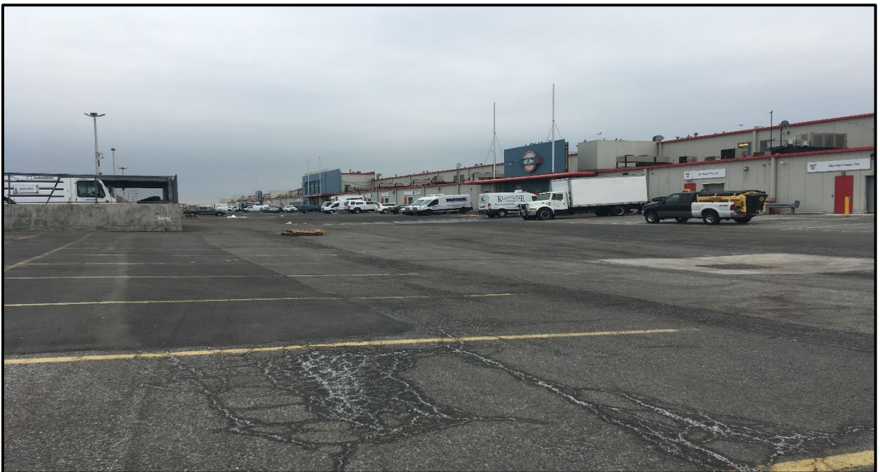
Photo 12: Facing south in the eastern portion of Site; engineering controls are still in place. Normal wear from heavy truck traffic in the form of asphalt cracks and potholes of various sizes are present in the parking lot (March 2019).
