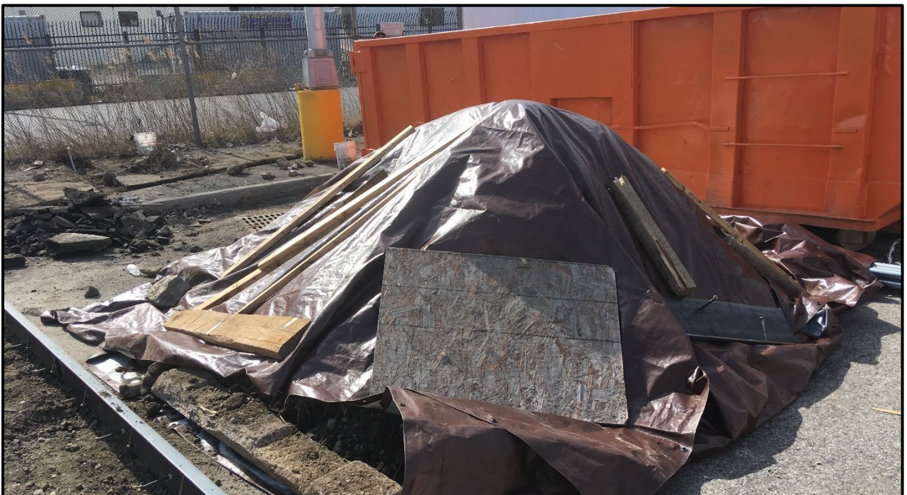
Photo 4: Facing northwest in the northwestern portion of Site; excavated soil on plastic sheeting and covered with a tarp to be sampled, characterized and disposed of at an appropriate facility (March 2019).
