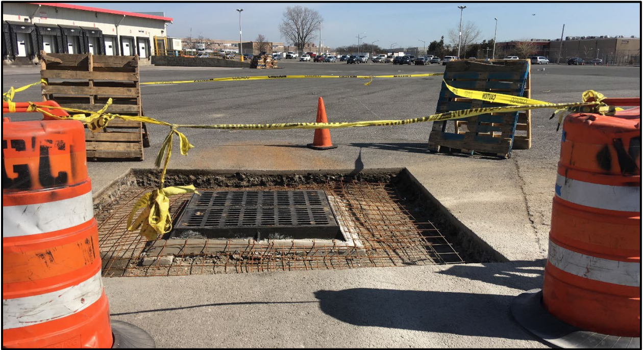
Photo 9: Facing east in the southern portion of Site; asphalt removed and subbase exposed for storm sewer drain repairs (March 2019).
