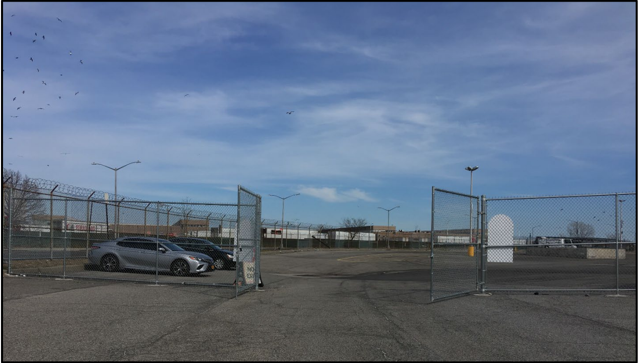
Photo 3: Facing east in the northeastern portion of Site; newly installed fencing and gated entryway completed by SH5 Construction Corp. (September 2018).
