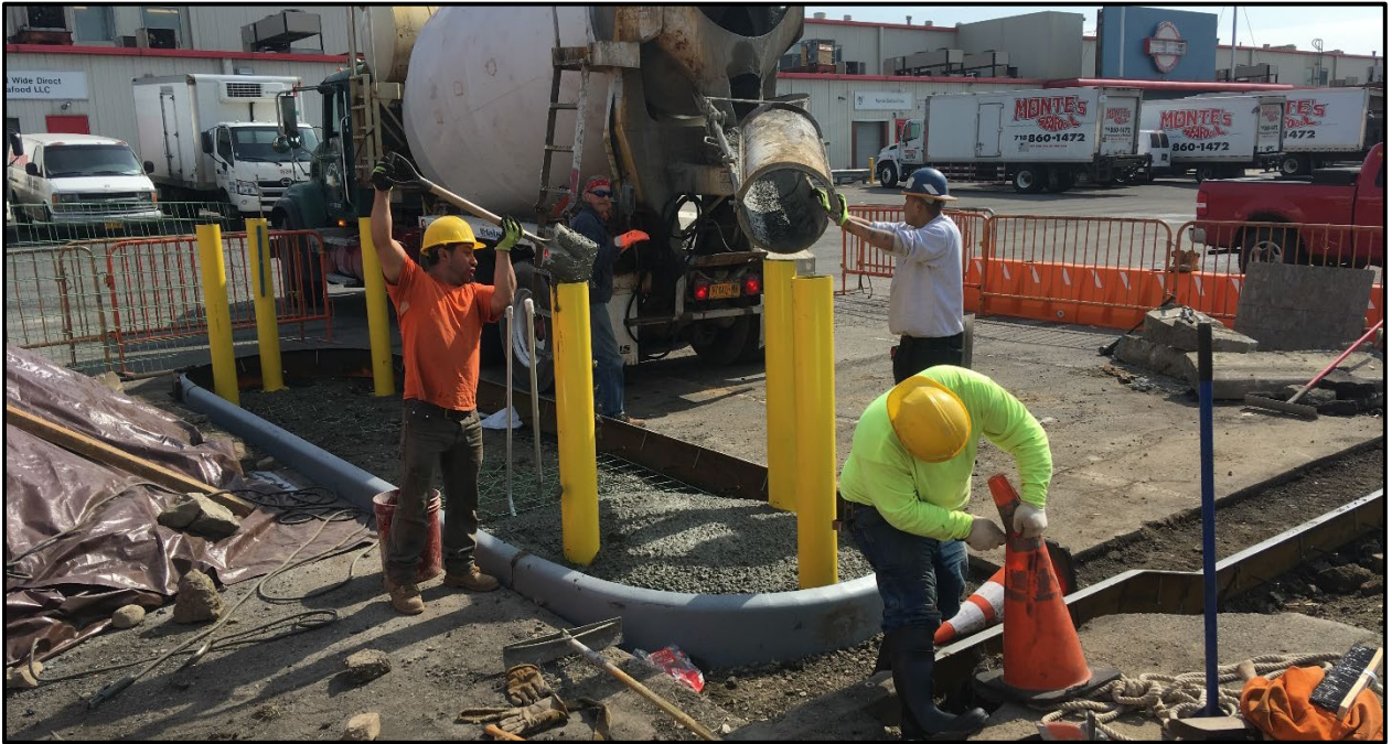
Photo 5: Facing east in the western portion of Site; Verdugos General Contractors Corp. pouring concrete for the guard shack foundation (March 2019).
