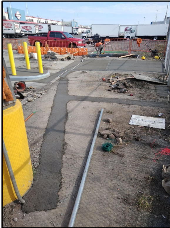
Photo 7: Facing south in the northwestern portion of Site; concrete poured over the electrical conduit trench, re-establishing the engineering cap (March 2019).
