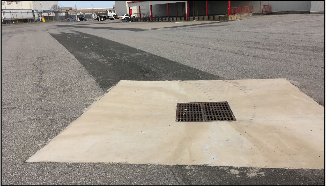
Photo 1: Facing east in the northwestern portion of Site; Storm sewer installation and re-paving/re-capping as performed by Verdugos General Contractors Corp. (mid-2018).
