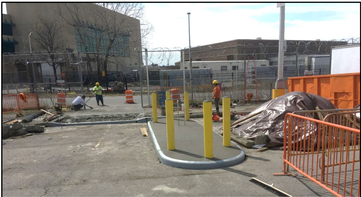
Photo 8: Facing west in the northwestern portion of Site; concrete poured over exposed subgrade material for the new guard shack foundation (March 2019).
