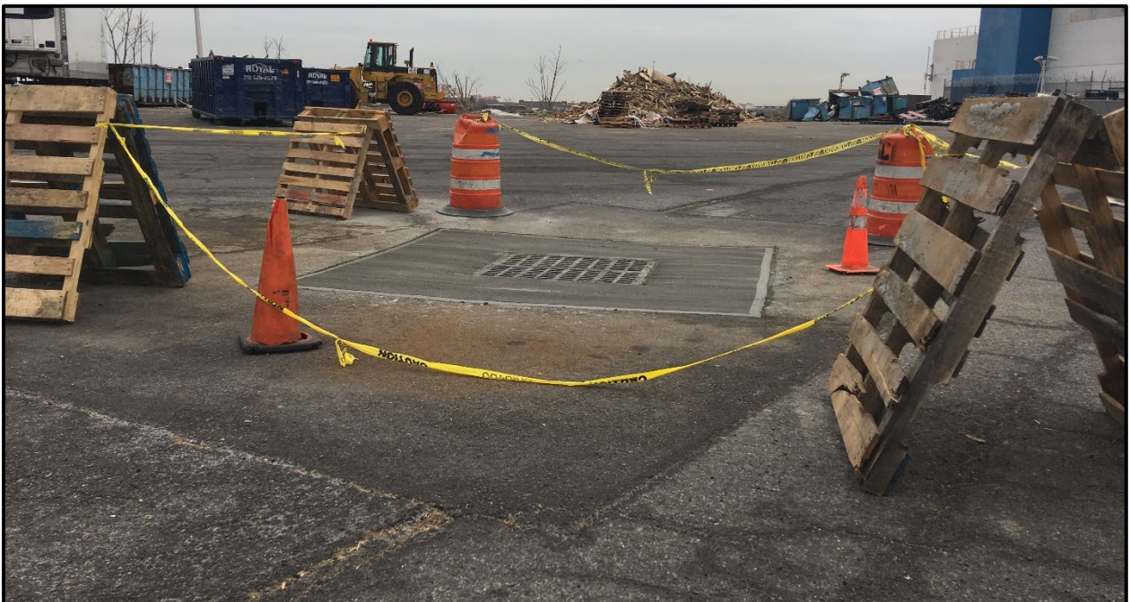
Photo 10: Facing west in the southern portion of Site; completed repairs on a storm sewer drain. Following the concrete pour, the EC was re-established (March 2019).
