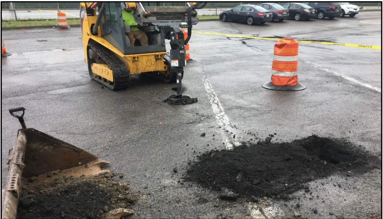
Photo 2: Facing northeast in the northeastern portion of Site; SH5 Construction Corp. augering holes for fencepost installation (September 2018).
