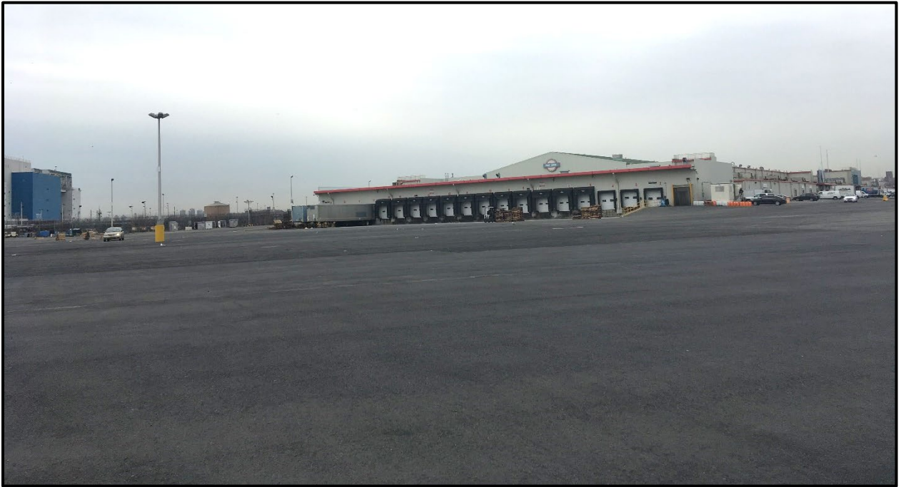
Photo 11: Facing north in the southern portion of Site; engineering controls are still in place. Normal wear from heavy truck traffic in the form of asphalt cracks and potholes of various sizes are present in the parking lot (March 2019).
