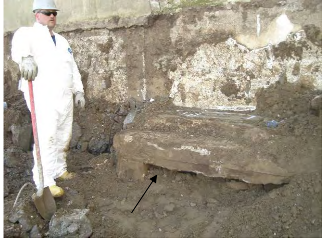
Site Restoration – Voids under retaining wall footing Void under Eastern Portion of Footing April 29, 2010
