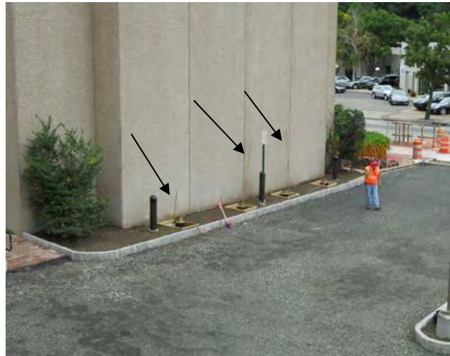
Site Restoration – Lighting Electrical Grounding Rods (not fully driven into ground) August 21, 2010
