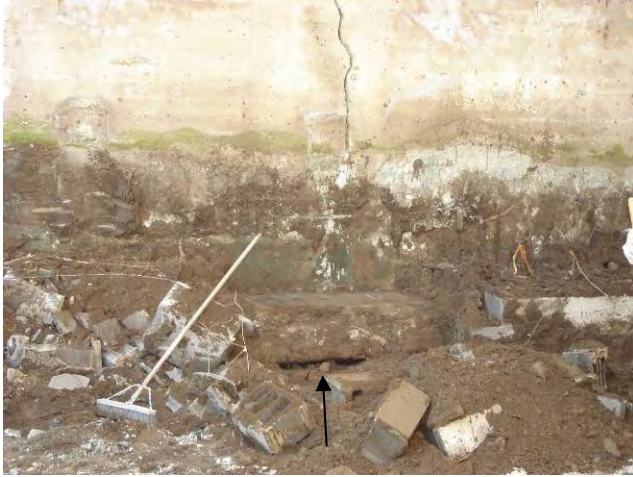
Site Restoration – Voids under retaining wall footing Void Under Central Portion of Footing April 29, 2010
