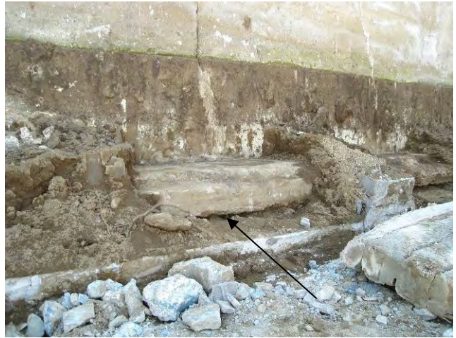
Site Restoration – Voids under retaining wall footing Void under Western Portion of Footing April 29, 2010
