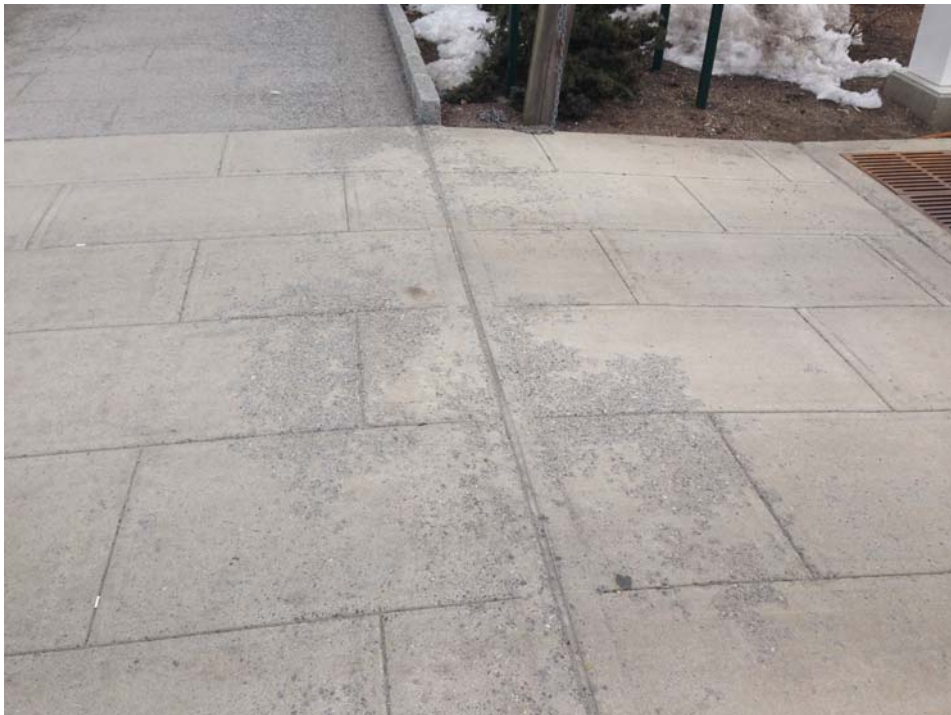
Photo 7: Spalling of Concrete in Sidewalk Near Northeast Entrance
