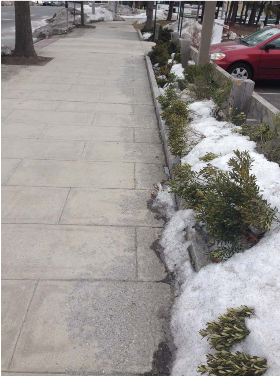
Photo 8: Spalling of Concrete along Water Street
