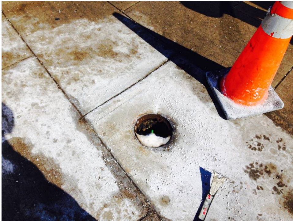
Photo 8: MW-18 Missing Cover on 3/6/15
