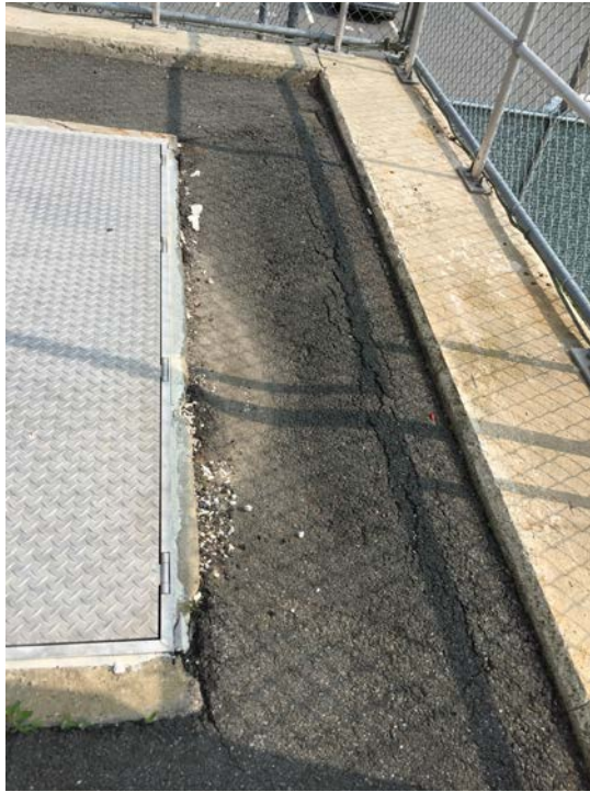
Photo 1: Substation Parking Lot depression along equipment vault (facing North)
