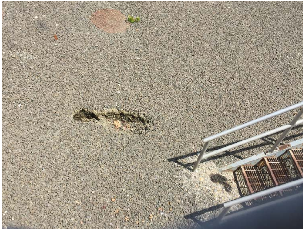
Photo 2: Sink hole in gravel cover area near Transformer Vault No. 3 (facing East)
