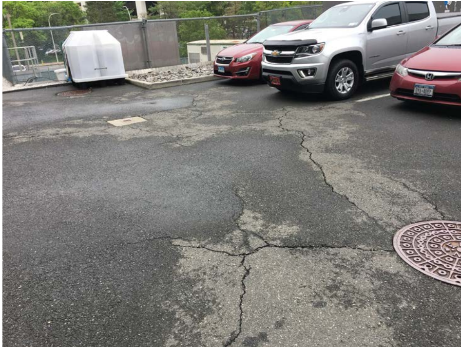
Photo 3: Substation Parking Lot (facing North)
