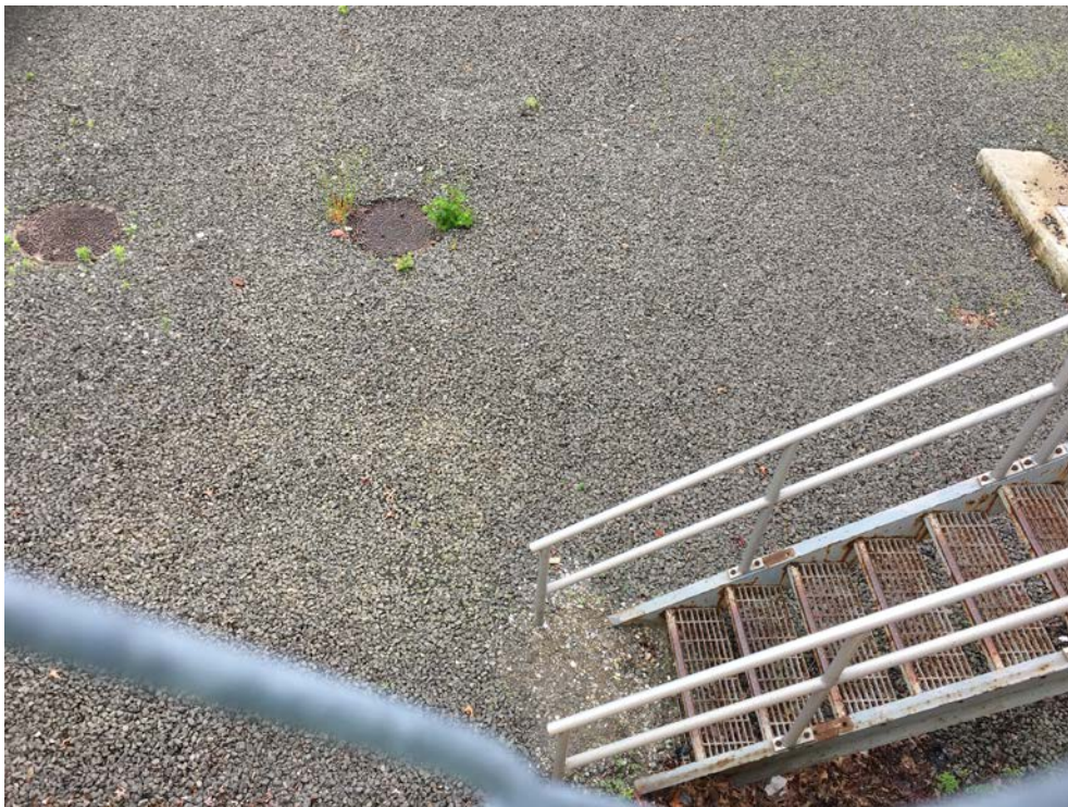
Photo 2: Sink hole no longer in gravel cover area near Transformer Vault No. 3 (facing East)
