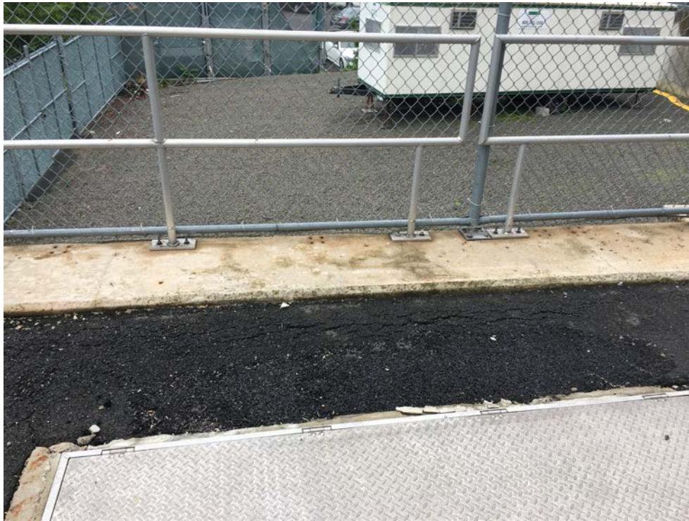
Photo 1: Substation Parking Lot equipment vault (facing East)
