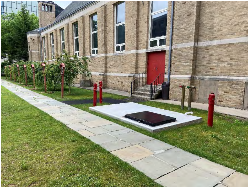
Photo 18: New Installed Tank for Fire Suppression
