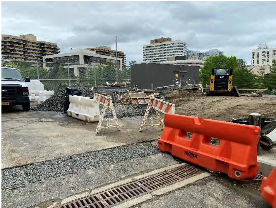
Photo 5: Substation Parking Area (Looking Northeast)
