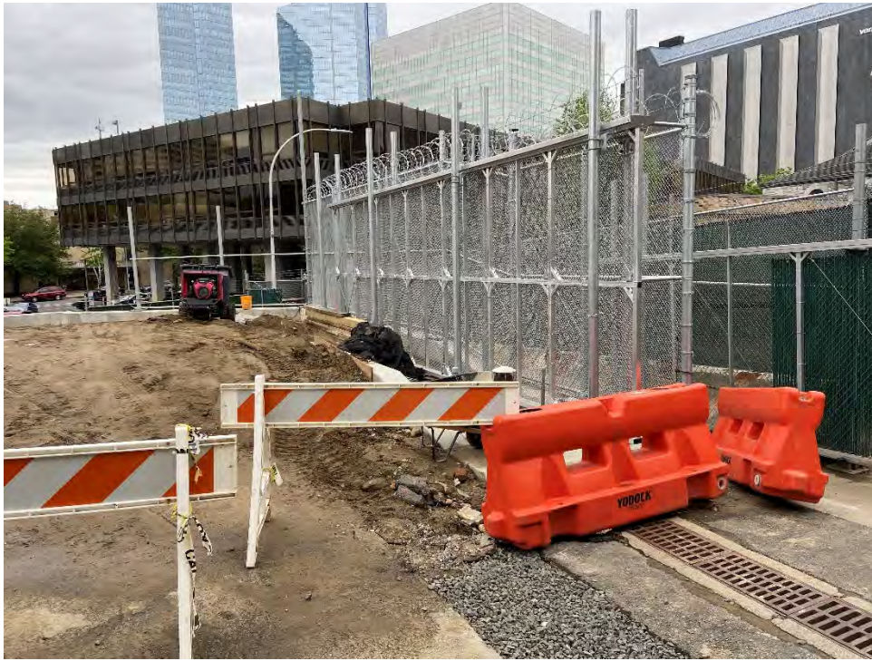
Photo 3: New Substation Slide Gate (looking Southeast)
