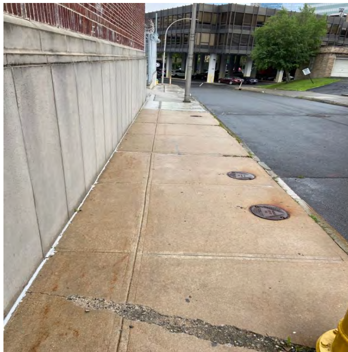
Photo 4: Recovery wells and monitoring well on the side walk (facing East)
