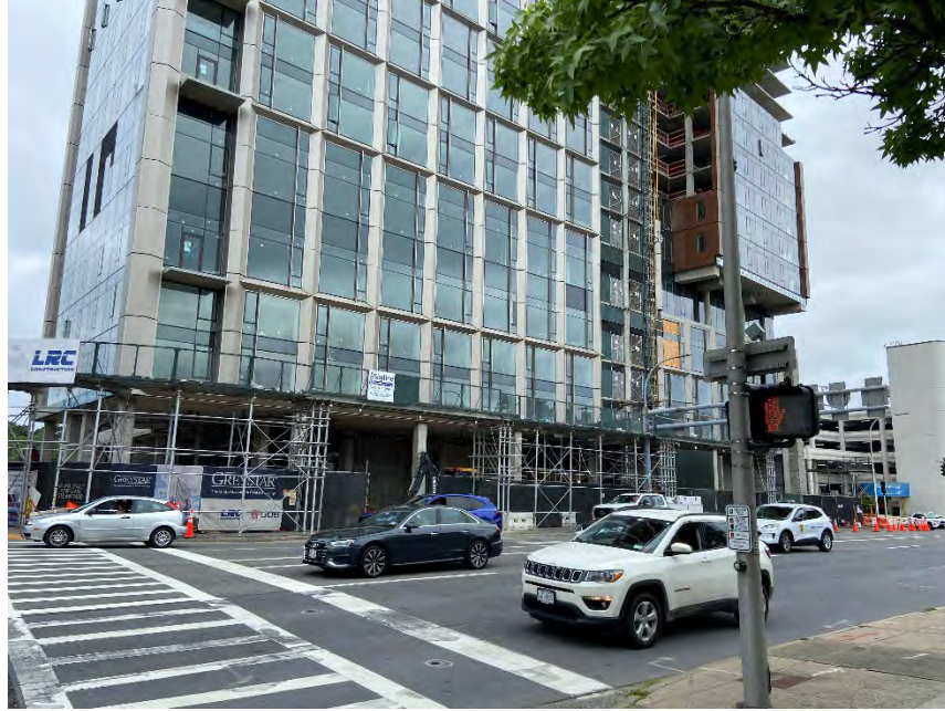
Photo 22: Building construction in progress across North Lexington Avenue from St. Johns western parking lot (facing Northwest)
