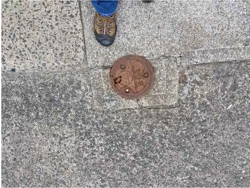
Photo 9: Monitoring Well MW-19 well cover is broken
