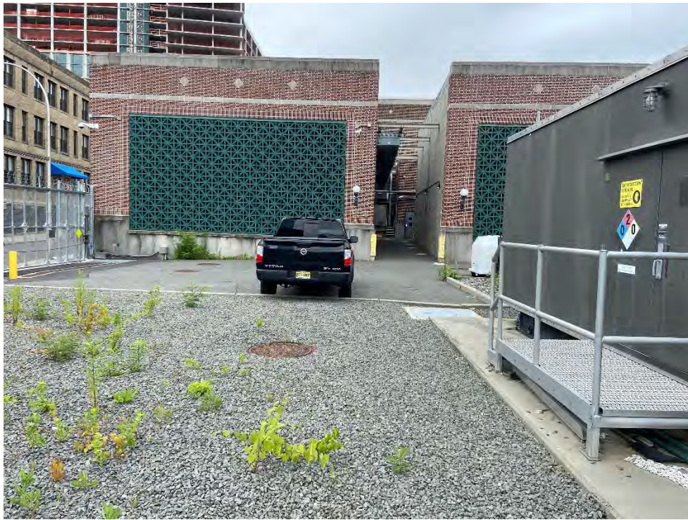
Photo 7: Upper gravel cover area near Transformer Vault No. 3 (facing West)
