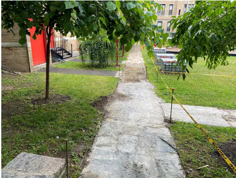
Photo 19: Preparation for surficial paver work in the St John's Courtyard (facing North)
