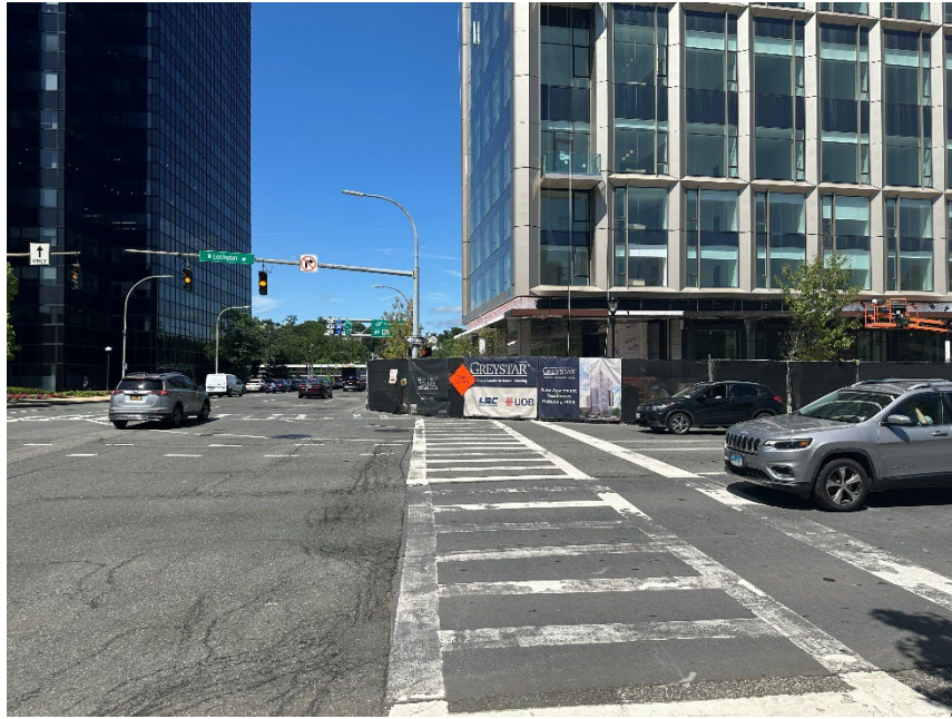
Photo 22: Building construction in progress across North Lexington Avenue from St. Johns western parking lot; MW-18 is behind construction fencing (facing Northwest)
