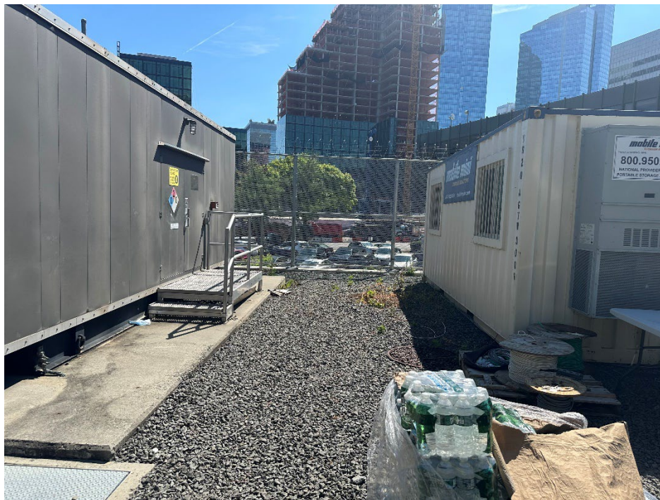
Photo 6: Upper gravel cover area near Transformer Vault No. 3 (facing East)
