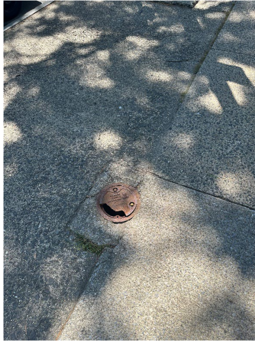
Photo 9: Monitoring Well MW-19 well cover is broken
