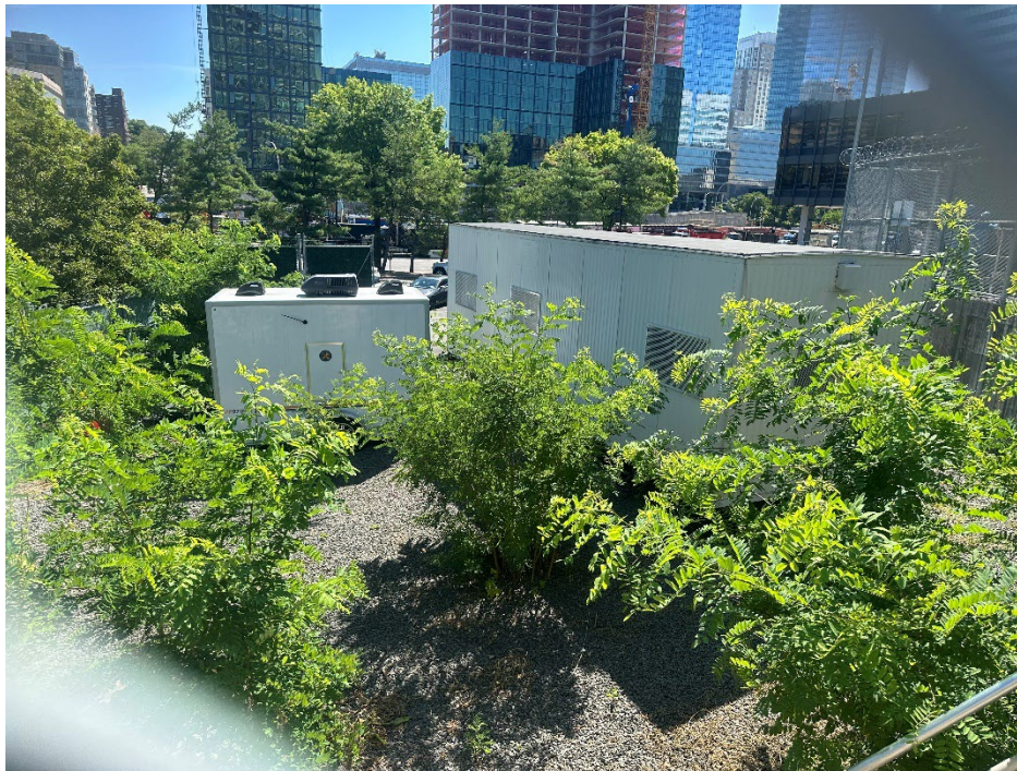
Photo 5: Lower gravel cover area near Transformer Vault No. 3 (facing East)
