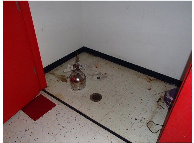
Photo 2: View of SS-103 installed in the basement of the former Tutor Time.
