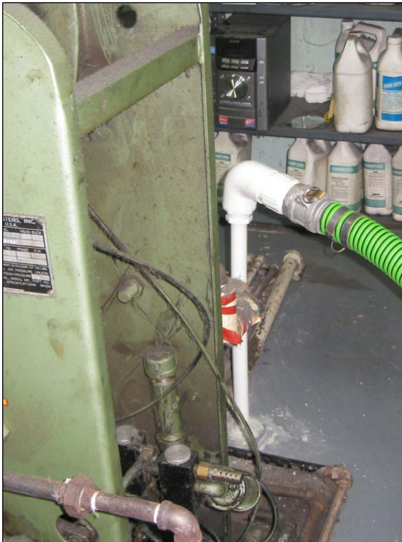
Photo 7. Connection of vacuum line from blower to extraction point XP2.
