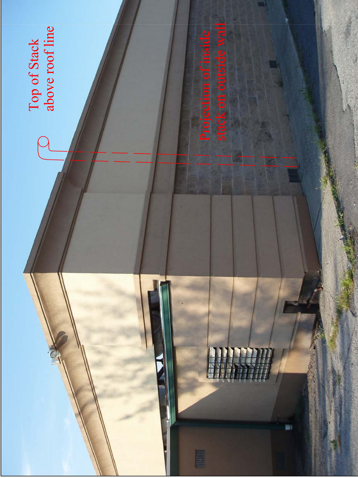
Figure 7. Outside left rear corner of building from backyard showing location of 4-inch PVC stack for Vapor Extraction System at American Cleaners at 360 Route 211 East, Middletown, NY 10940 NYSDEC DER VCP V-00461-3, September 2012
