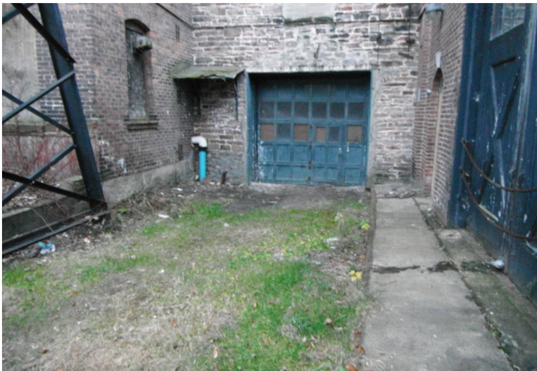
OF-06 (continued): Source of the pipe that comes from the building, runs under driveway, and extends through retaining wall by the river.
