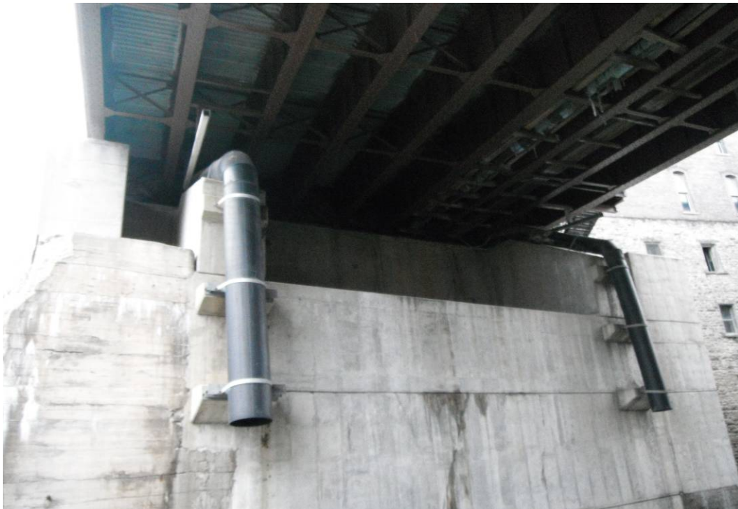
GP-12: View of two 24" diameter pipes on west side of river under Main St. Bridge. The distance between the two is roughly 45'. Pipes apparently drain storm water from roads/parking lots.
