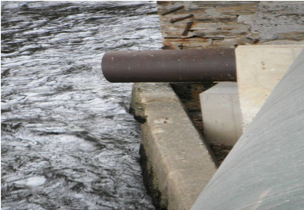
GP-11: Picture of the other 18-24" metal pipes under bridge on east side of river.
