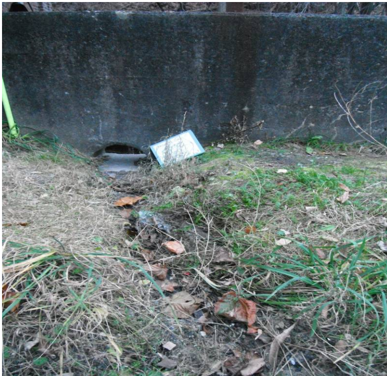
OF-07 (continued): Distant view of OF-07. Notice makeshift channel to promote drainage toward hole.
