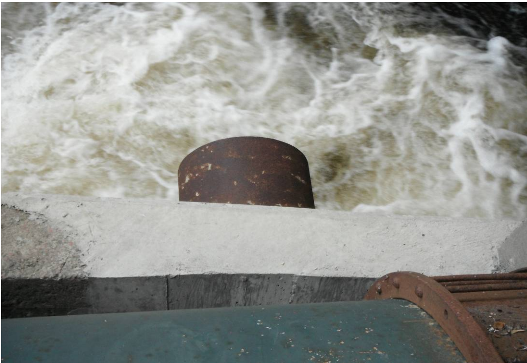
GP-10: Picture of one of the two 18-24" metal pipes under bridge on east side of river.
