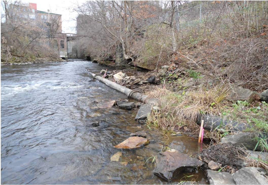
GP-01: West side of bank looking upstream of Salmon River, site immediately to the right. Survey stake in lower right corner is NG-SR-SD-05. The view is of the municipal sewer pipe with the tar patty area extent in the background. The downstream extent of patty is upstream from NG-SR-SD-05, approximately 5 – 10' and just west of the pipe. Note the power-generating building on the east side of river, in the background.
