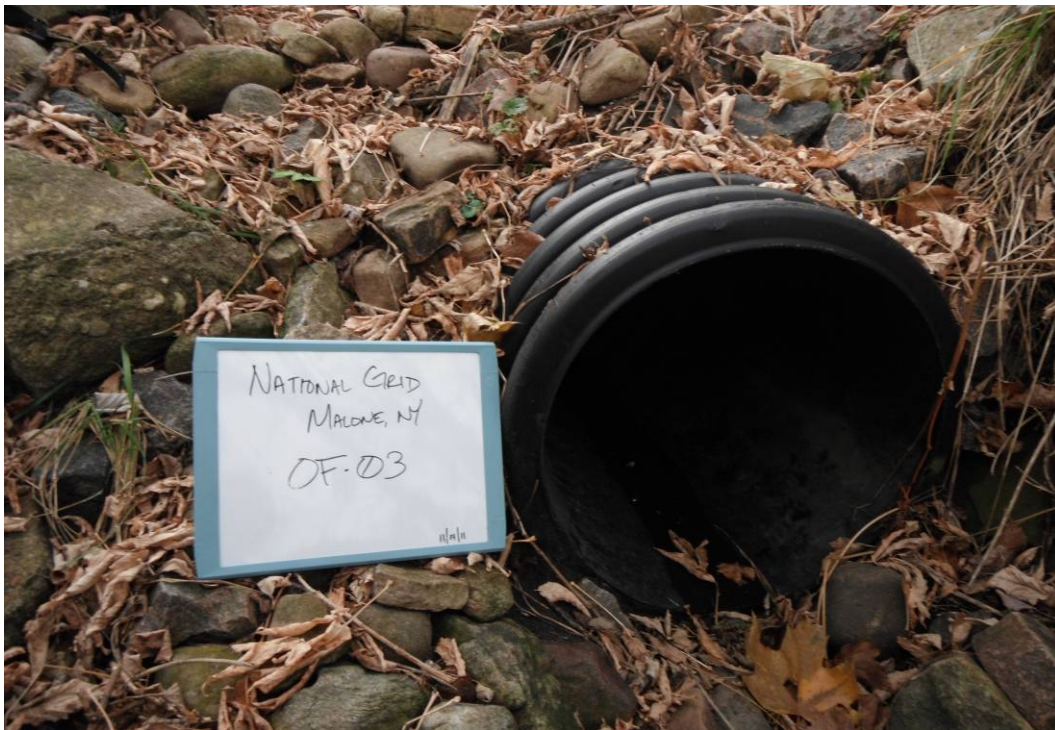
OF-03: 18" HDPE pipe on west side of river. The pipe is about 30' from the riverbank, roughly 10' higher than river elevation, and approximately 200' upstream from bridge. Approximate 10 mL/min discharge observed at time of photo.
