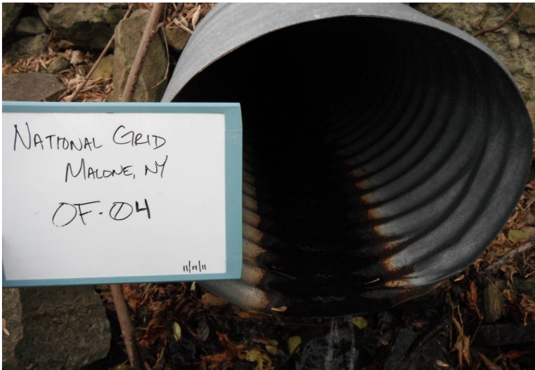
OF-04: 24" CMP on west side of river. Pipe is approximately 5-10' from the river bank, about 5' higher than river elevation, and roughly 100' upstream from bridge. A discharge rate of approximately 1000-1500 mL/min observed at time of photo.
