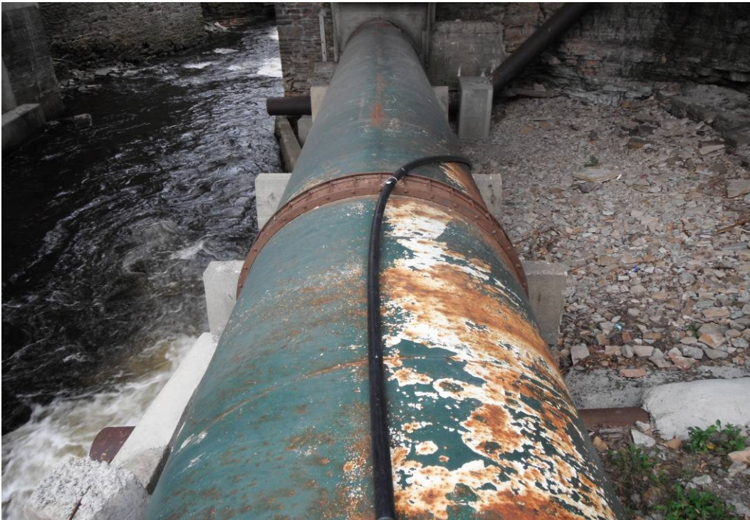
GP-09: Large (8' - 10' diameter) power-generating feeder pipe. Notice that pipes from photo GP-08 run underneath the municipal pipe and into river.
