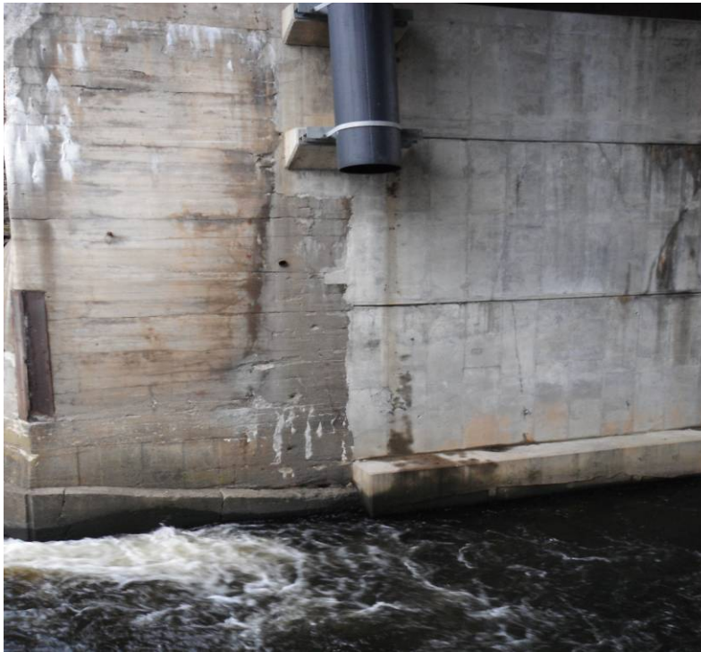
GP-13: Picture of the more upstream of the two 24" metal pipes under bridge on west side of river. Notice two small 3-4" metal pipes coming out of retaining wall just left and slightly below large pipe.
