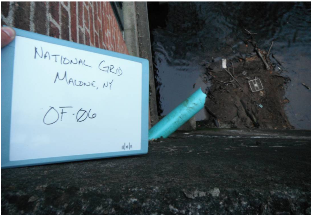
OF-06: 8" PVC pipe on east side of river. Power generator building immediately left on photo. The pipe is approximately 30' above river elevation. Large sediment deposit below is location of NG-SR-SD-16. No discharge observed from pipe at time of photo.
