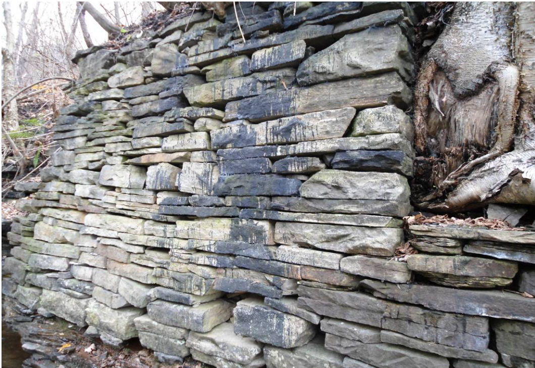
GP-05: Tar drips down foundation wall of former powerhouse on western riverbank of site, immediately upstream from tar patty. Survey point NG-SR-SD-02 borders the southern (upstream) side of the rock wall.
