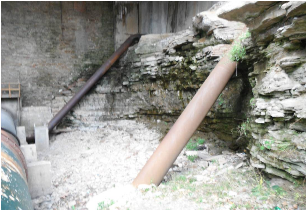
GP-08: 18-24" diameter metal pipes on east side of river under Main St. Bridge. Pipes go up and over exposed bedrock and under the large feeder pipe to power generator building. The pipes are about 60' apart from each other.
