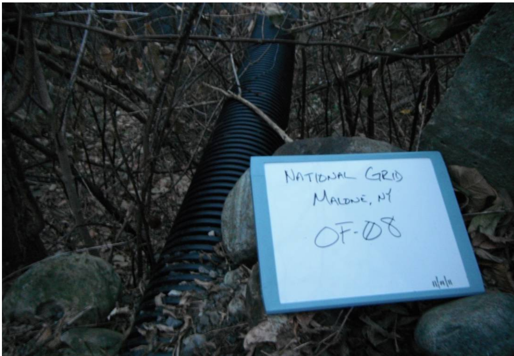
OF-08: 10" HDPE pipe on east side of river. The pipe is about 30' higher than river elevation and about 15' from river's edge.
