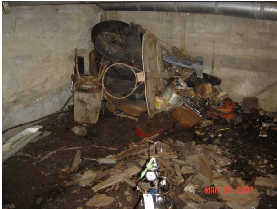
Photo 6 Basement of the Residence at 2 King Street Miscellaneous Debris (Old Tires, etc.) in the Southeast Corner
