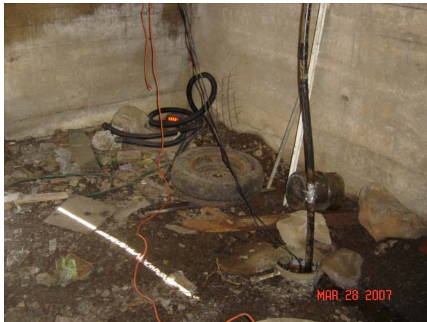
Photo 7 Basement of the Residence at 2 King Street Sump and Miscellaneous Debris in the Northwest Corner
