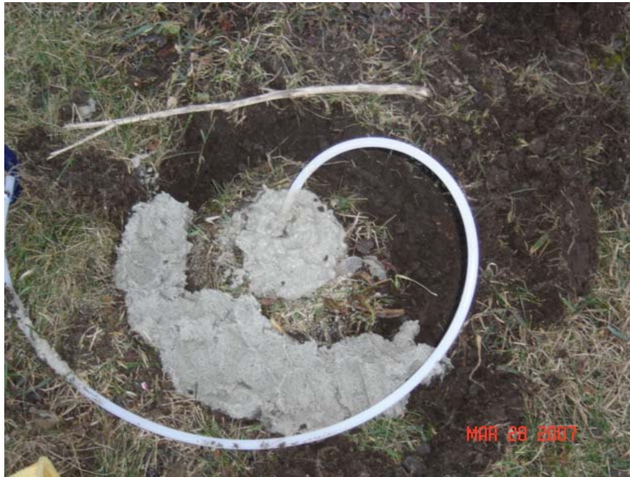
Photo 1 Sampling Location VP-1A Sample Point Installation – Adjacent to 2 King Street
