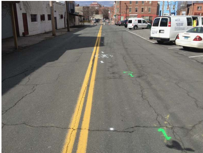
View along Hill Street to the northwest. Southern tar well to extreme lower right of photograph. White paint marks feature trend and assumed paved-over manhole. Green paint marks broken 6-inch clay pipe originating near southern tar well.
