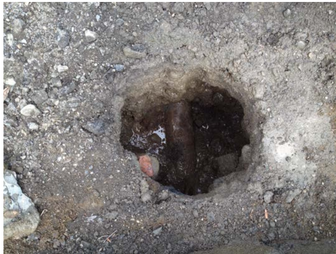
Gas main found near center of Hill Street in TP-1-13
