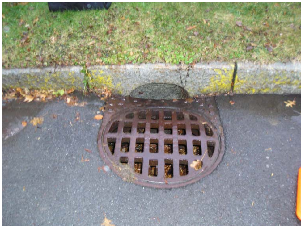
Photograph #1 –Washington St. catch basin (CB#1) for storm water flow. Substantial amount of debris within catch basin, unable to determine flow direction, if any. Top of photo is northeast.
