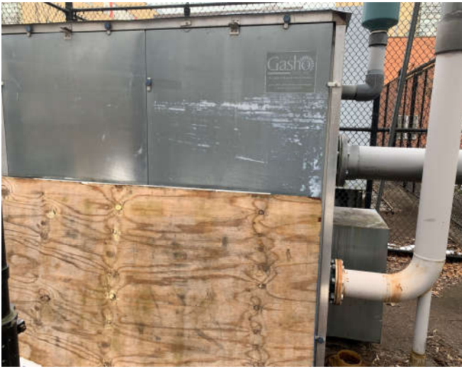
Photo 1: View of the SSDS unit on the exterior.
