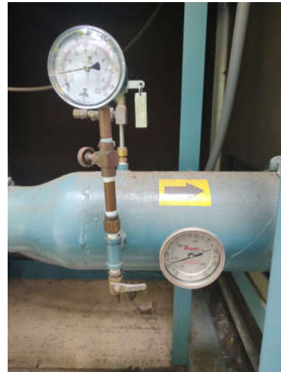
Photo 2: View of blower outlet pressure.
