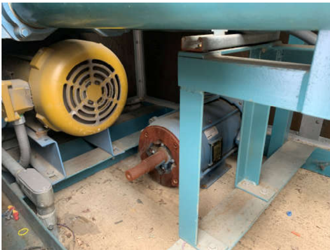
Photo 3: View of the SSDS fan motor.
