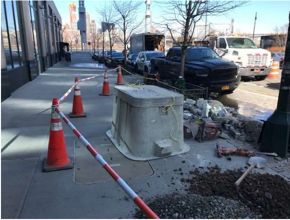
Photo 9. Junction box (facing north).
