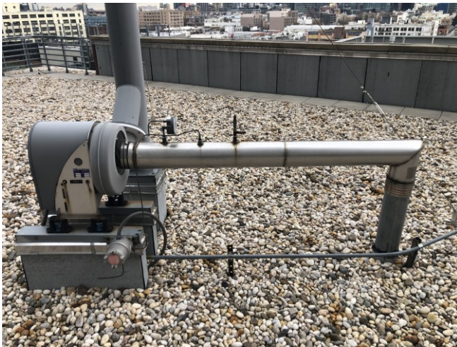
Photo 3: View of SSDS fan unit SSDS-1.
