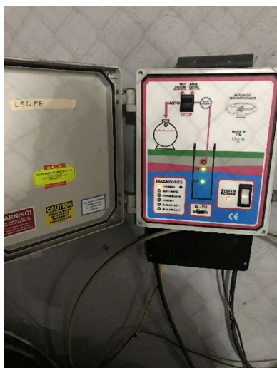
Photo 23: Control panel for LNAPL recovery well L56PE inside of 45-45 Center Blvd. (C241095)
