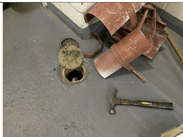
Photo 25: Typical SSDS monitoring point cover
