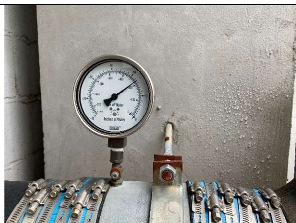
Photo 27: Typical SSDS pressure gauge confirming operation of SSDS blower at 46-30 Center Blvd. (V00505B)
