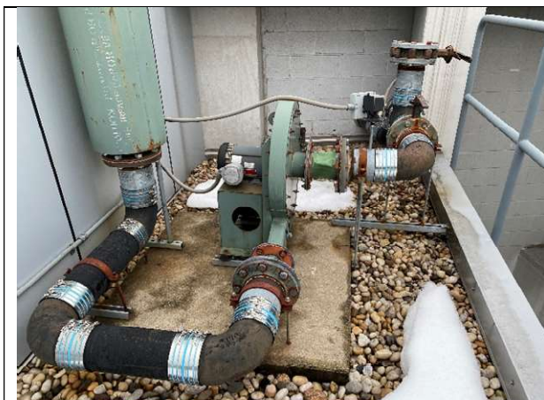
Photo 21: View of SSDS blower fan and on the roof of 46-30 Center Blvd. (V00505B)
