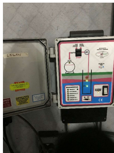
Photo 24: Control panel for LNAPL recovery well L56PN inside of 45-45 Center Blvd. (C241095)
