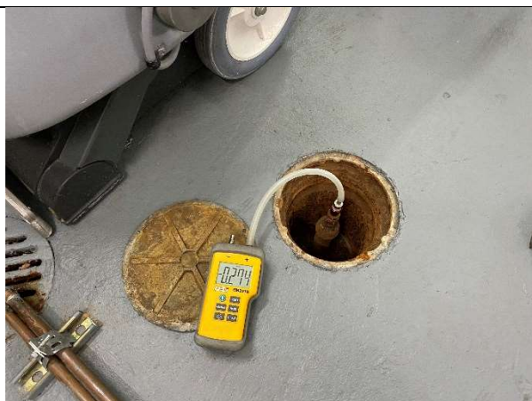
Photo 26: Typical SSDS monitoring point measurement tap
