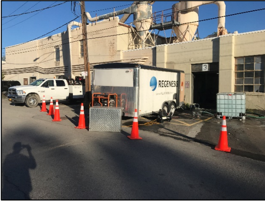
Photo 1: RRS injection trailer on-site.
