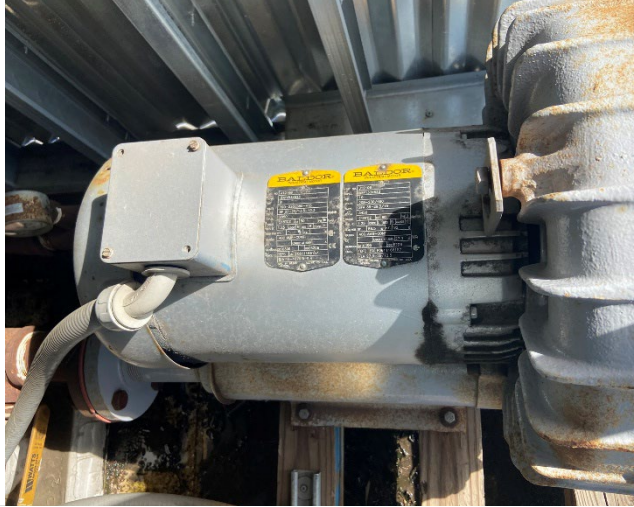
Blower #2 specification placard (9.26.25)
