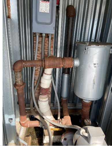
Blower #2 enclosure interior (9.26.25)
