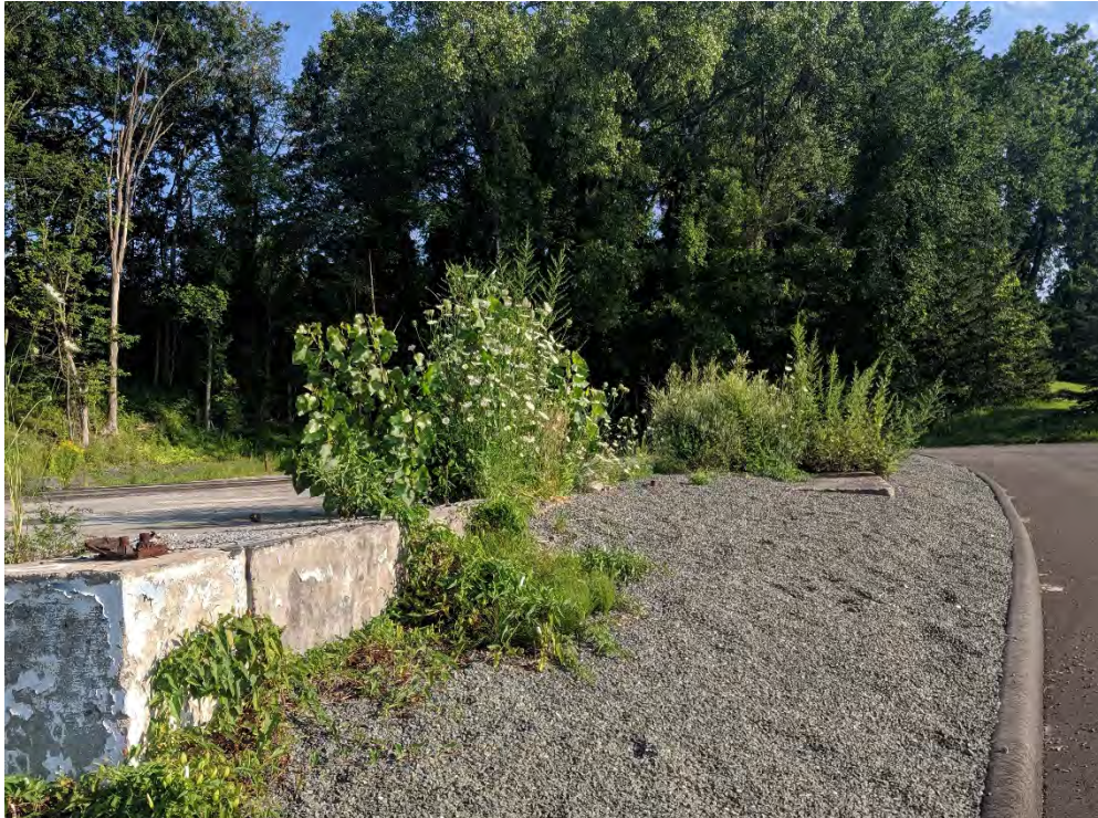
Photo 7: Stone cap condition before vegetation removal (facing south).
