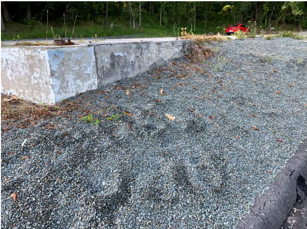
Photo 8: Stone cap condition after vegetation removal (facing southeast).
