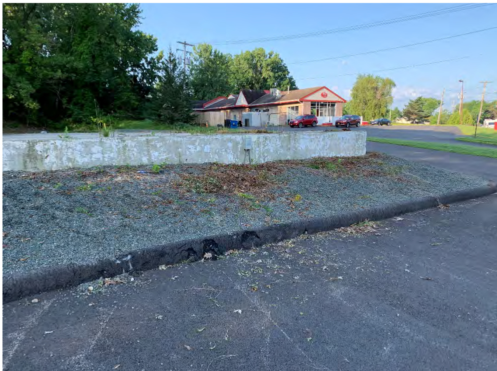
Photo 6: Stone cap condition after vegetation removal (facing south).
