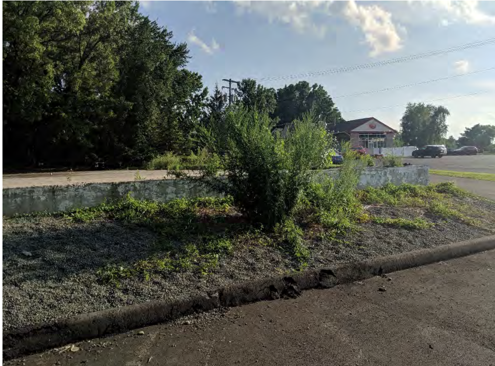
Photo 5: Stone cap condition before vegetation removal (facing south).
