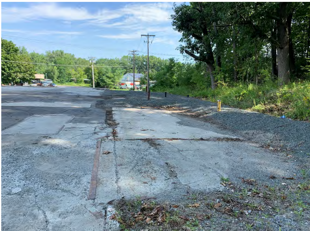
Photo 6: Concrete cap condition after vegetation removal (facing north).
