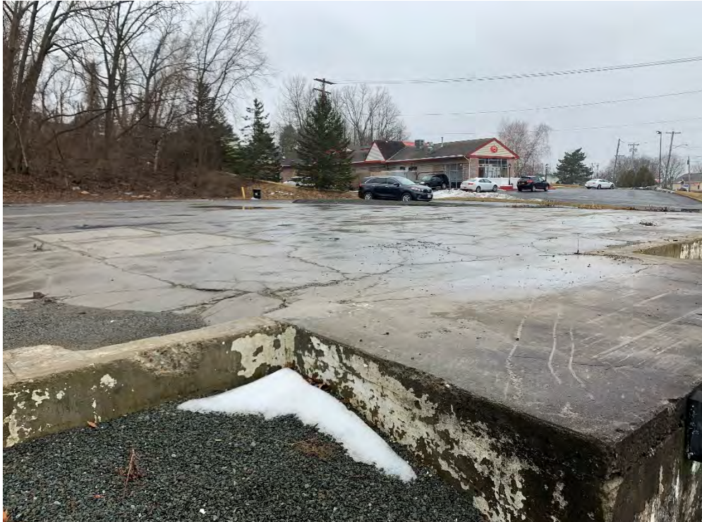
Photo 3: Concrete cap condition (facing southwest).
