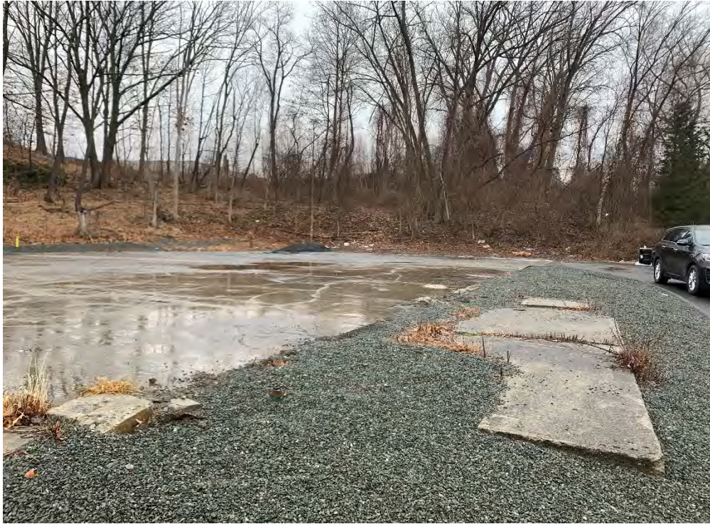
Photo 5: Concrete and stone cap condition (facing southwest).
