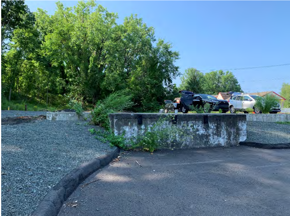
Photo 3: Concrete cap condition prior to vegetation removal (facing south).
