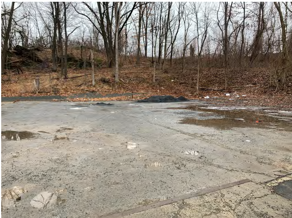
Photo 2: Concrete cap condition (facing southeast). Note small pile of stone in southeast corner.
