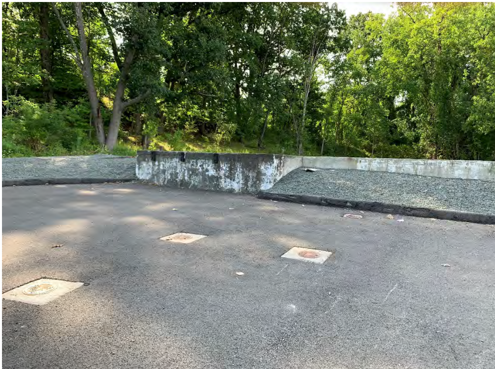
Photo 4: Concrete cap condition after vegetation removal (facing southeast).
