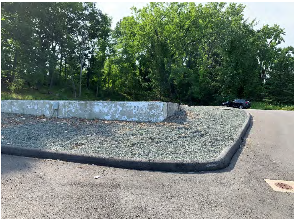
Photo 2: Concrete cap condition after vegetation removal (facing southeast).
